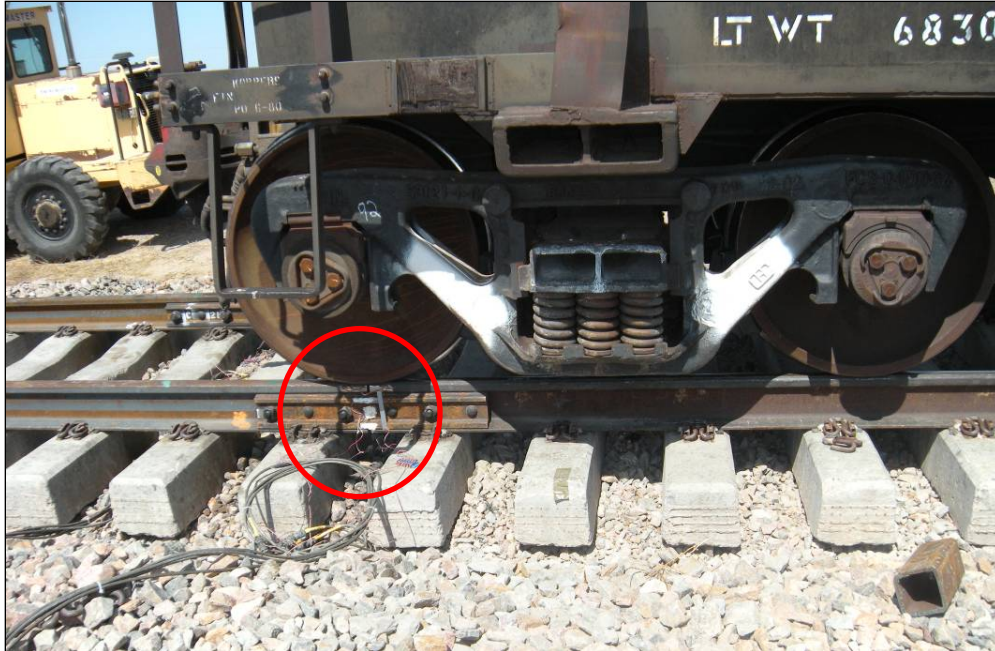
Figure 5. Car Wheel on the Joint Center during Static Data Collection (photo shows joint with disturbed foundation)
