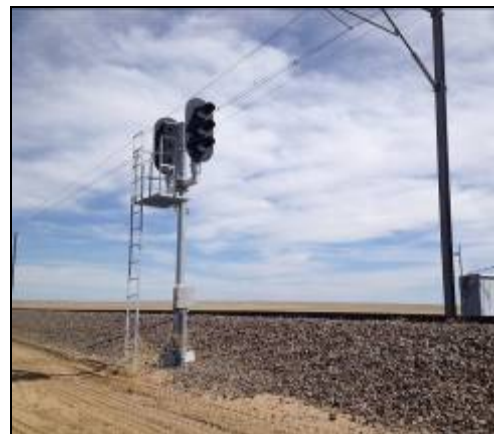
Figure 1. Railroad Test Track Block Signal Light
