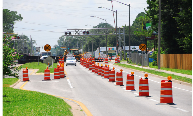
Orange drums guide drivers through this work zone. Each drum is required to have retroreflective sheeting and a warning light.
