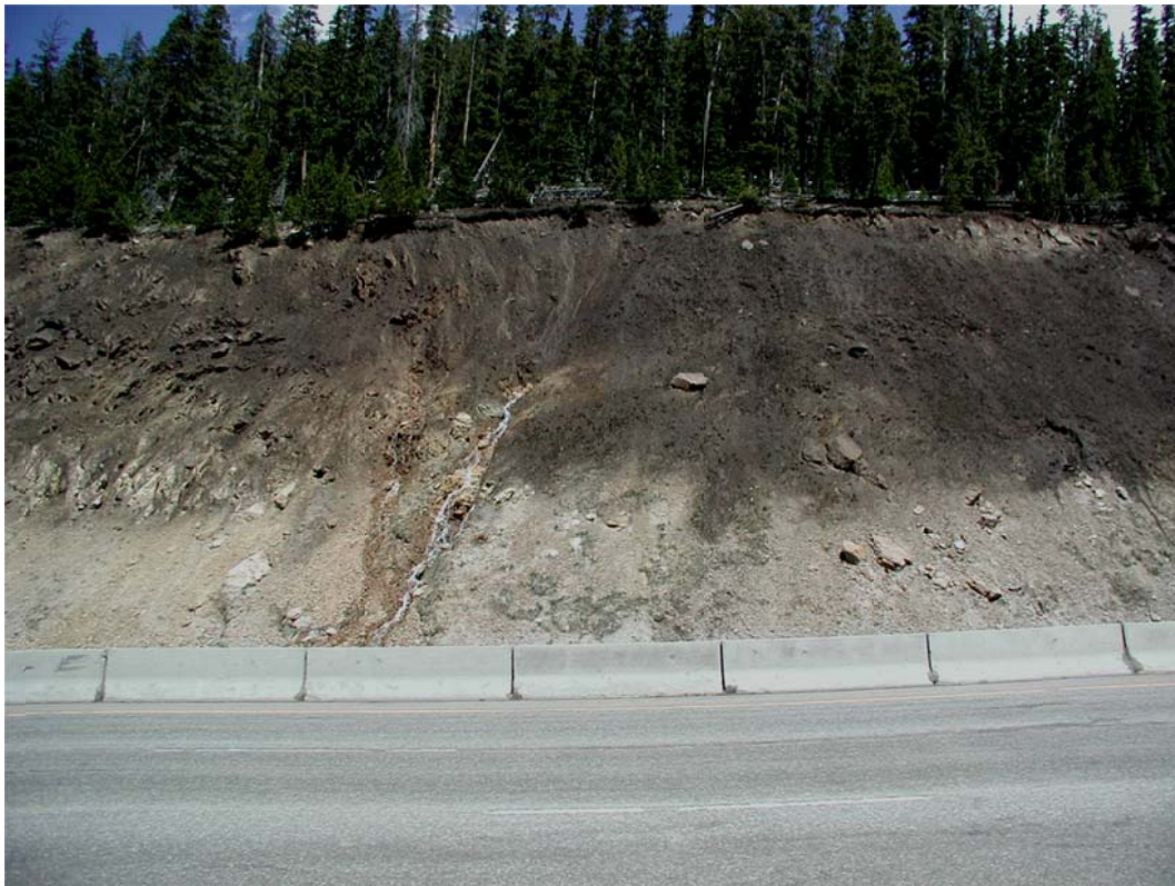
Figure 1. Unvegetated slope soon after construction before erosion control and revegetation treatment (T. Weldon, CDOT photo).
