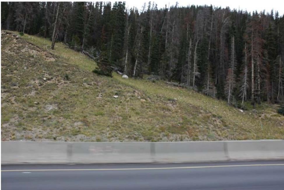
Figure 2. Native soil plots N1 and N2 on the shallow slope of a graded access ramp running from center right to upper left. There was native soil on this area of the site, although it had been disturbed by grading. Plot N1 was located behind the conifer on the slope edge and plot N2 was located just left of the dead snag at the slope edge in the upper left of the photo. Revegetation plots V5 and V6 are located on the cut-slope face just below the single conifer at the slope edge, as delineated by rows of stakes on the plant transect ends and the plot corners. Photo from 2008.
