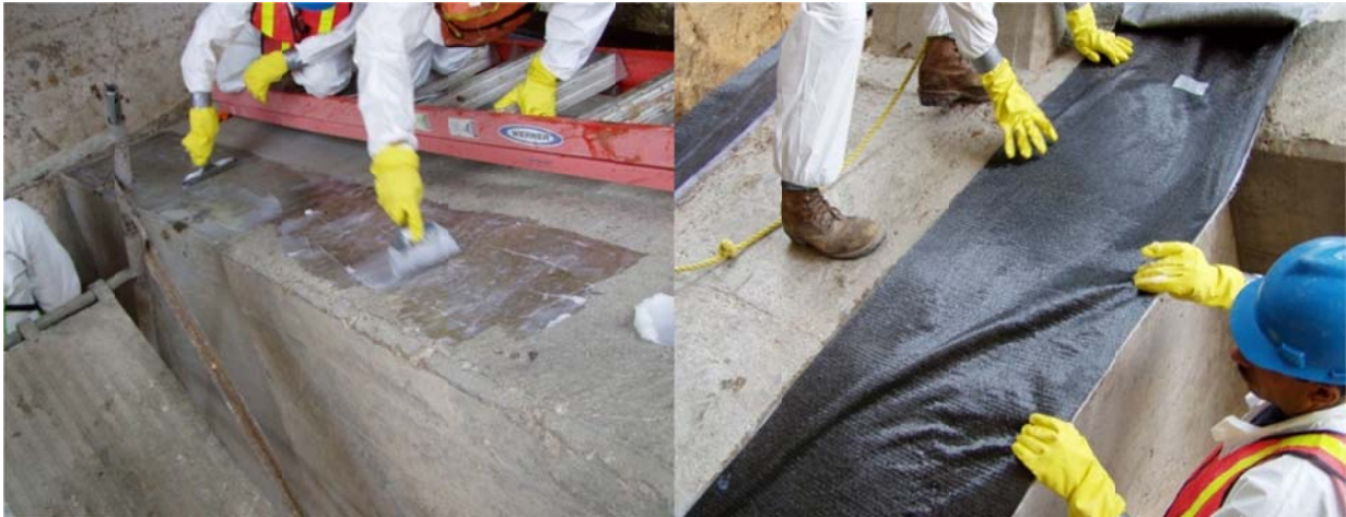
Figure 2.10. Fyfe’s Tyfo® S Epoxy resin (likely with glass fibers as a filler) being applied to the extrados of an arch and installation of saturated unidirectional CFRP fabric, Tyfo® SCH-41 (Mohseni, CDOT)
