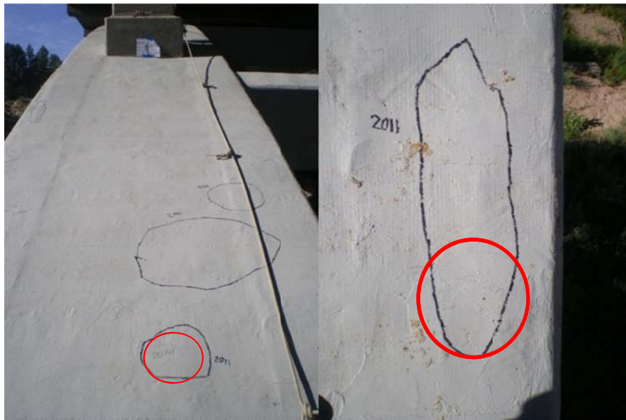
Figure 2.14. Outlined in permanent marker are identified areas of debonding between the FRP and the substrate developed in the structure between inspections in 2007 and 2011. Faintly denoted in the bottom of the photographs (enclosed in red circles) are previously found voids identified with “DELAM 07” and lines distinguishing the boundaries of the voids.
