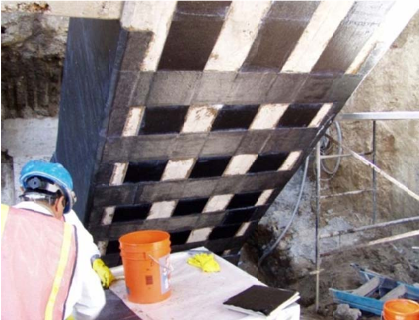
Figure 2.11. Longitudinal and transverse CFRP wraps at the base of an arch (Mohseni, CDOT)
