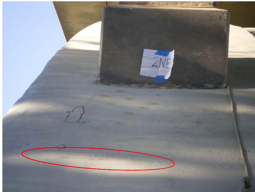
Figure A8. Previously identified in 2007, a crack enclosed in the red oval, no debonding at the location of the crack
