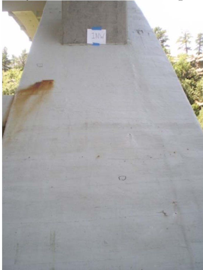
Figure A1. Bay 1NW, 2 of the 3 small voids and rust spot
