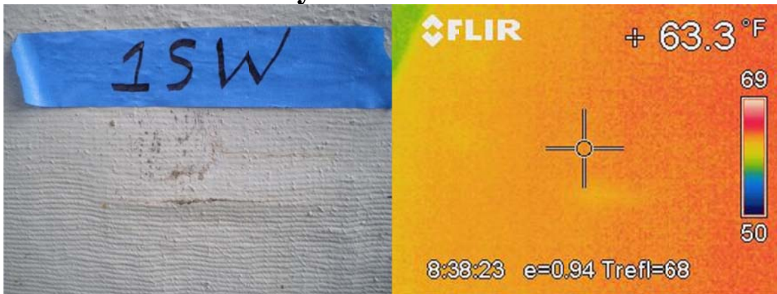
Figure A24. Photograph and thermal image of a defect found in Bay 1SW
