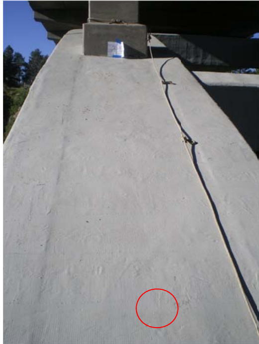
Figure A9. Bay 3NE with 1 of the 2 defects found in 2007 shown
