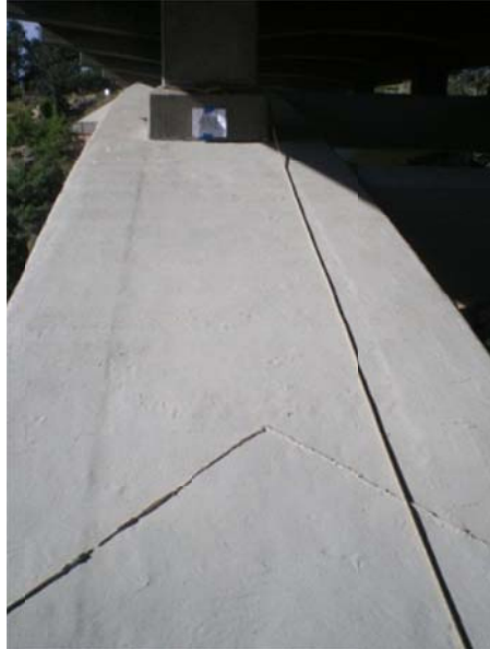
Figure A13. Bay 4NE, V-shaped silicone bead water diverter
