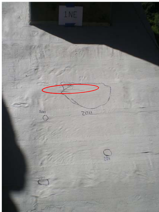
Figure A4. Bay 1NE, 4 of the 5 voids; crack exists, enclosed in red oval, in the top of the largest void
