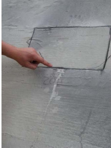
Figure 3.21. Water exiting the void area directly after the lower cut through the CFRP was completed
