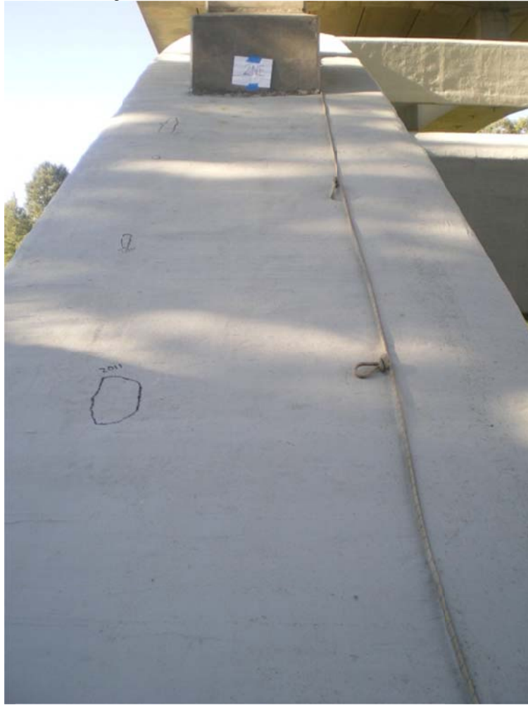
Figure A6. Bay 2NE, 3 voids
