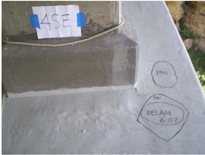
Figure 2.15. Enclosed in permanent marker are identified areas of debonded areas between the FRP and the substrate from 2011 and June, 2007. Notice in this more protected bay of the structure the markings from 2007 are more clearly visible.
