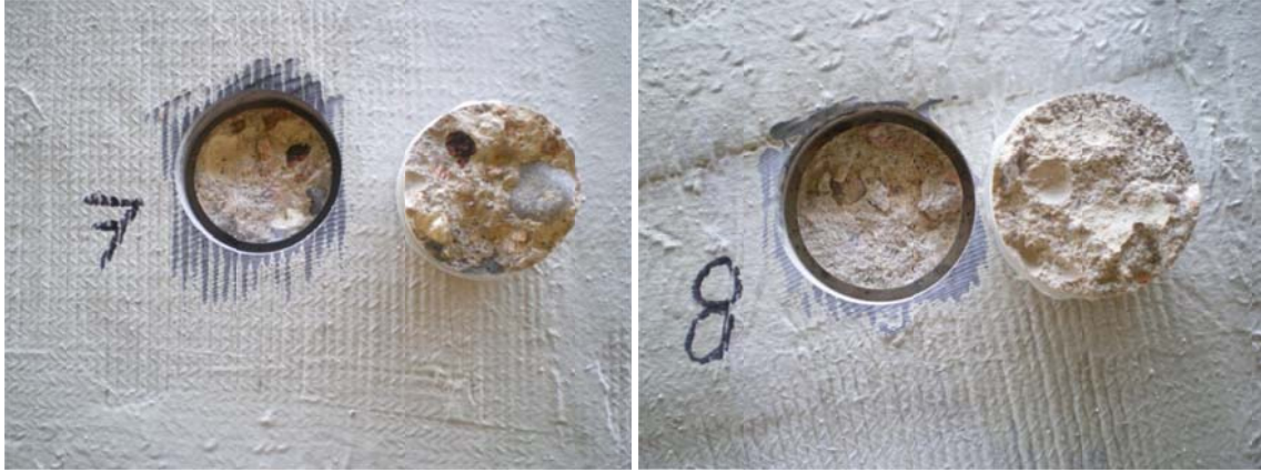
Figures B22 and B23. Test No.25 and test No.26, note very weak bond strength (poorly mixed concrete?)
