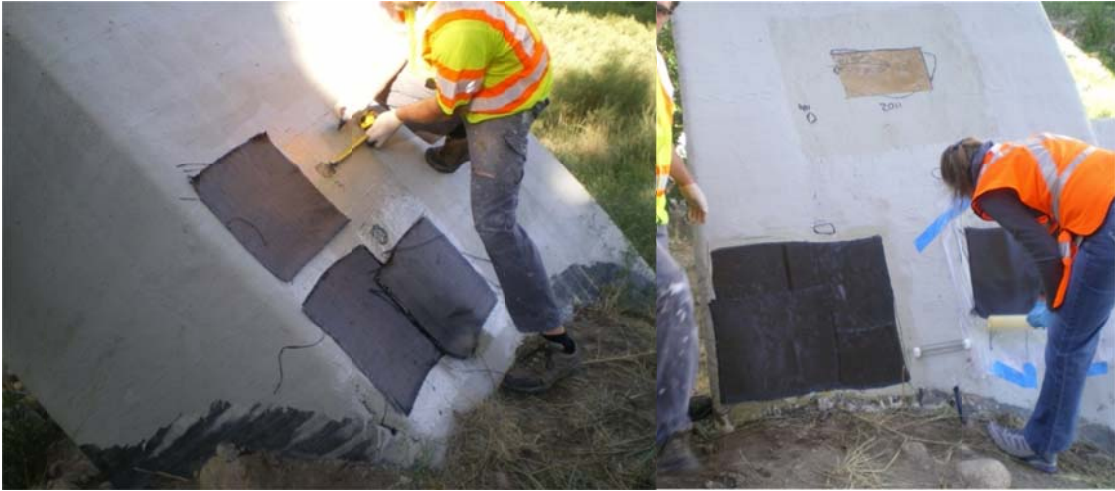
Figure 3.26. Allocating fabric for repair and applying the second layer of CFRP to the area of pull-off tests on the east arch
