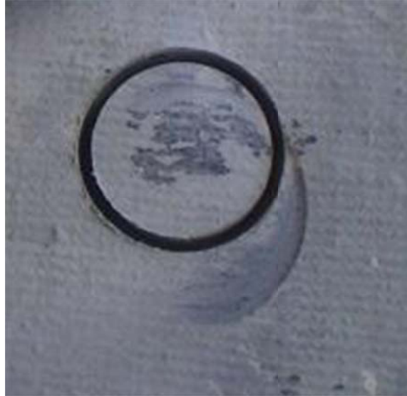
Figure 3.4. Damage caused by core bit without the use of the jig
