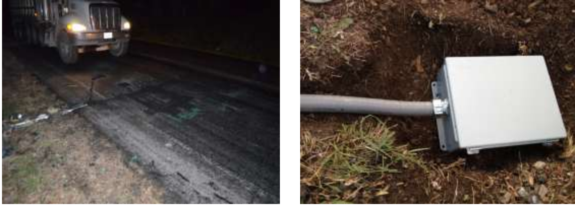
Figure 8: Installation Procedure (a. marking, b. cutting, c. paver passing, d. output cable management)
