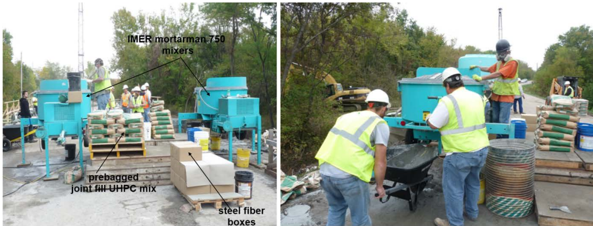
Figure 81. Photos. Batching of UHPC joint fill using IMER Mortarman 750 mixers in field.
