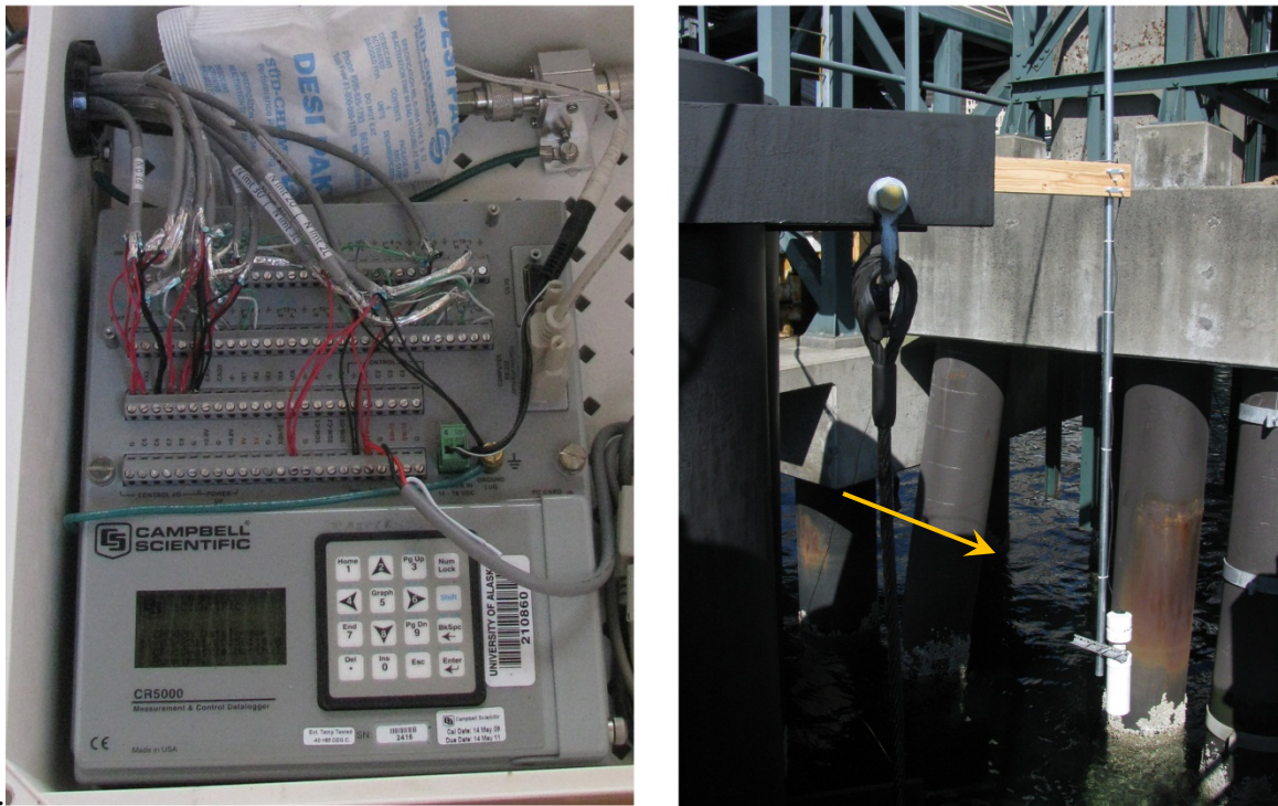
Figure 3.42: Datalogger and distance sensor photos. Datalogger (left) wired with wingwall instrumentation; distance sensor (right) measuring the tide elevation.
