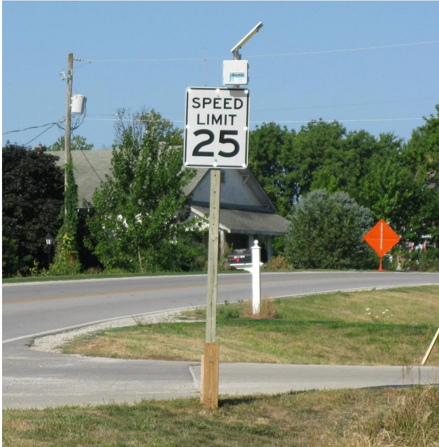
Figure 3-12: Radar-activated LED speed limit sign
