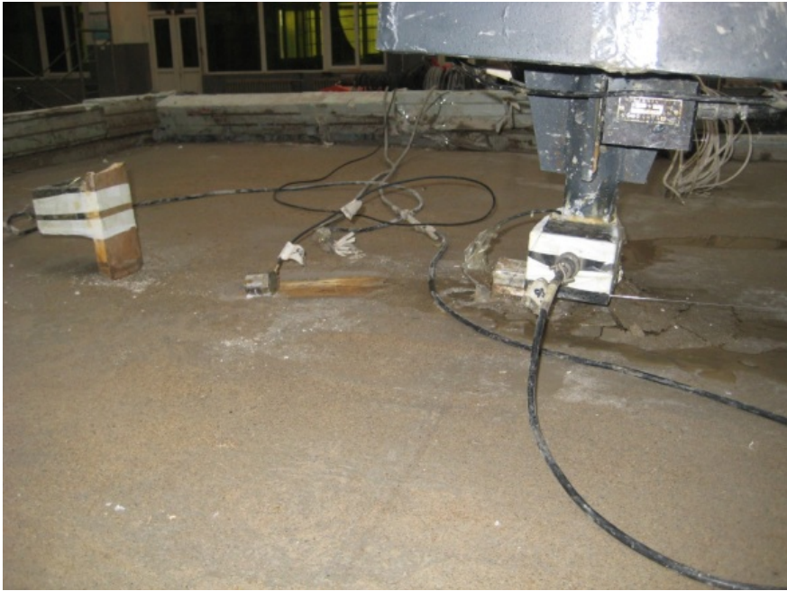
Figure 2.17. Tilted pile head
