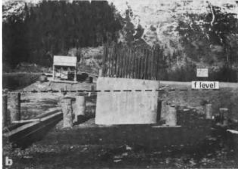
Figure 1.3. Ground settlement and tilted bridge pier at a bridge construction site
