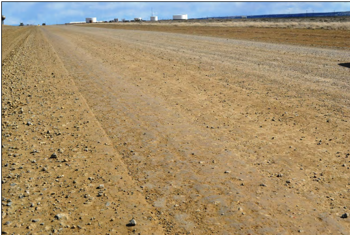
Figure 4.32 Road surface made of limestone crushed base treated with magnesium chloride on Sweetwater County's Crooks Gap Road.
