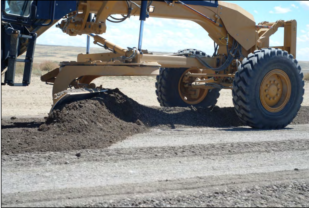
Figure 3.32 Blending and shaping the existing aggregate and CTB blend on Sweetwater County's Crooks Gap Road, August 2010.
