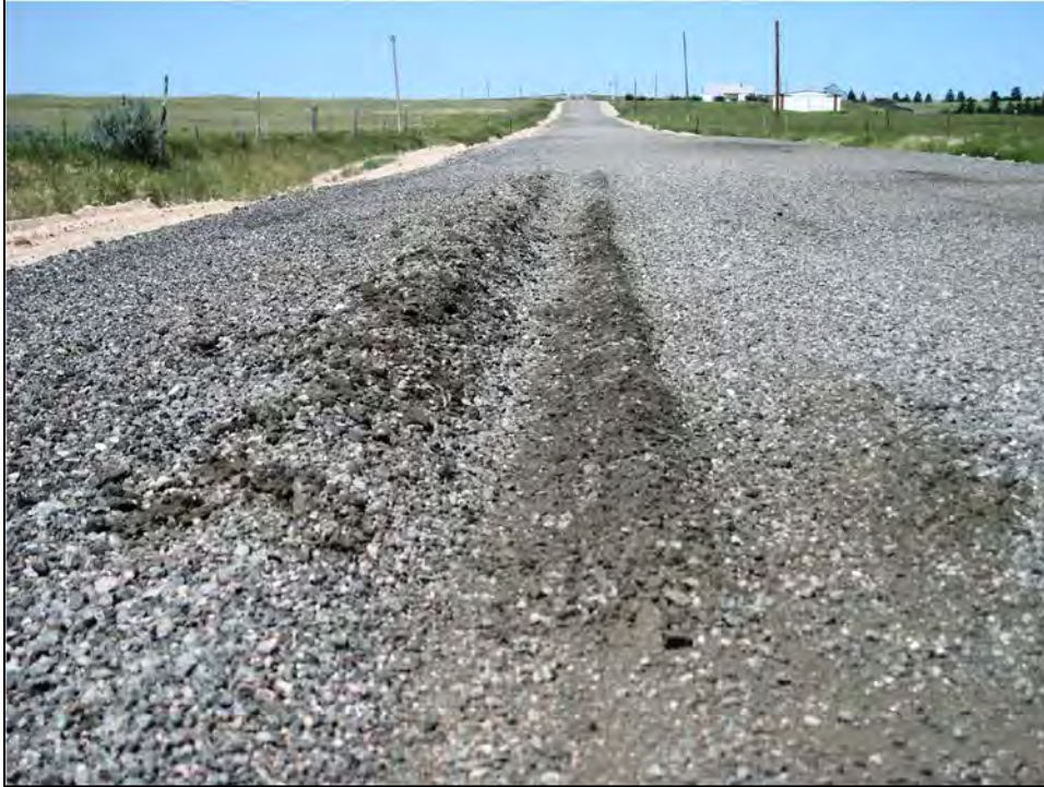
Figure 4.12 Nearly 100% RAP resulting in excessive loose aggregate on Laramie County's Atlas Road in June 2008, about two months after initial application.
