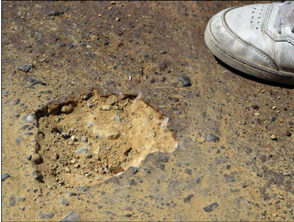
Figure 4.36 Crust formed by application of lignin and magnesium chloride dust suppressant applied to limestone crushed base on segment C of Sweetwater County's Crooks Gap Road in August 2011, three weeks after application of dust suppressant.
