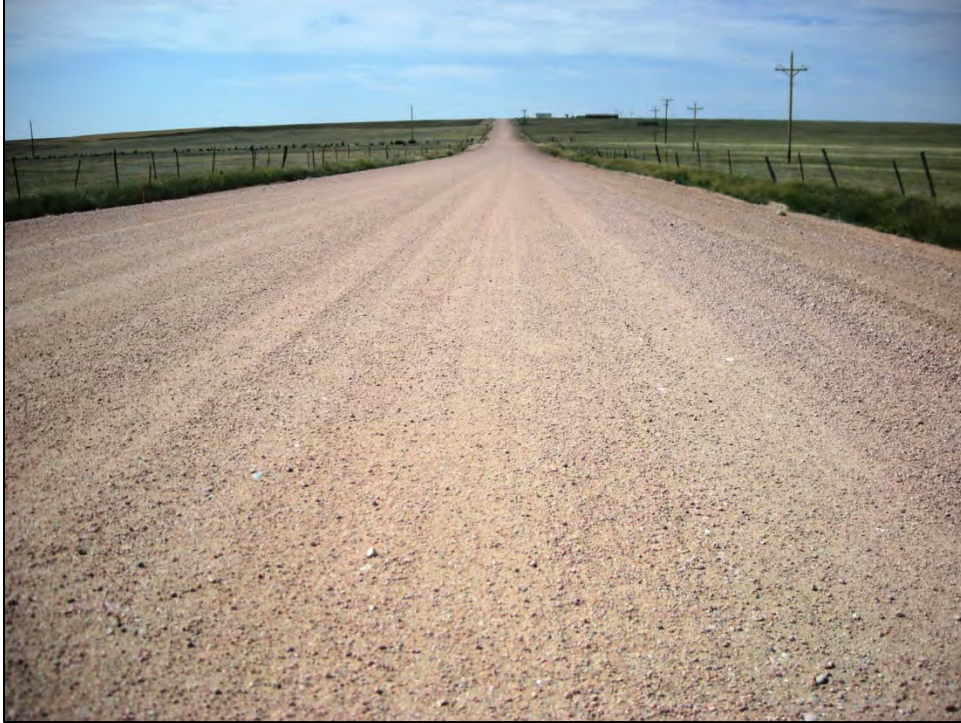
Figure 4.17 Aggregate only forming a good driving surface on Laramie County's Pry Road in July 2008, two months after shaping.
