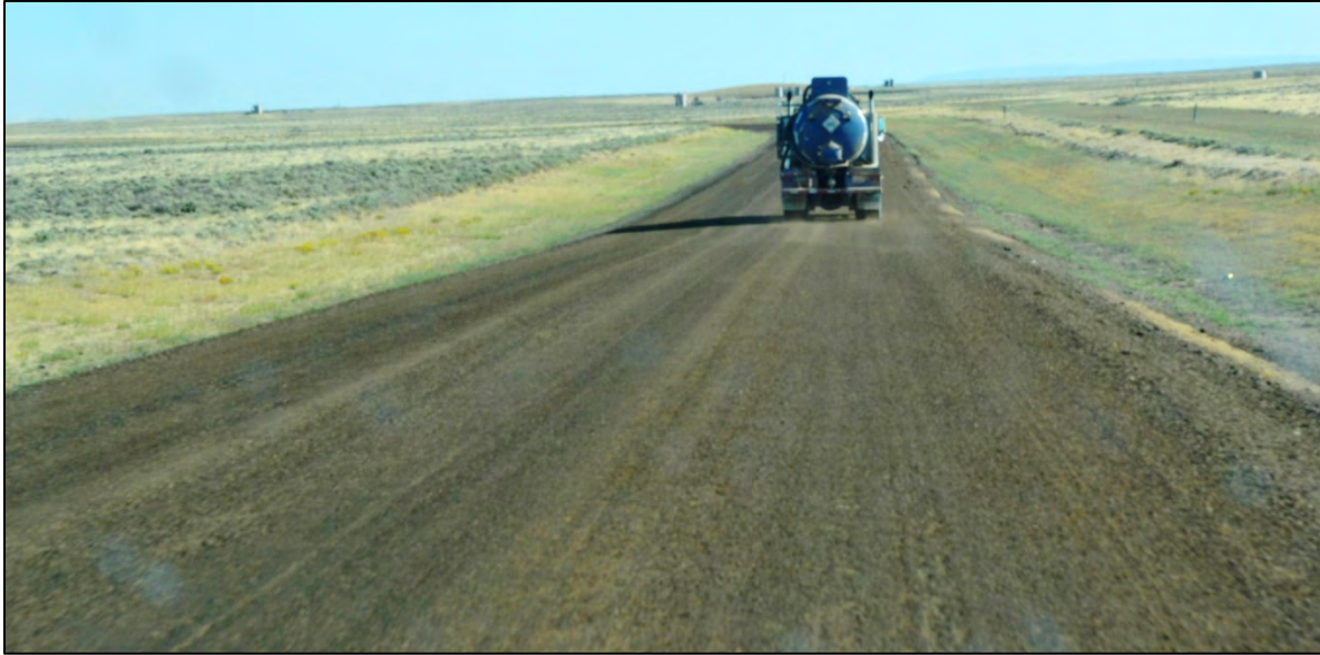
Figure 4.47 Road surface made from RAP blended with existing aggregate treated with magnesium chloride and polymer on segment M of Sweetwater County's Crooks Gap Road in August 2011, three weeks after application of dust suppressant.
