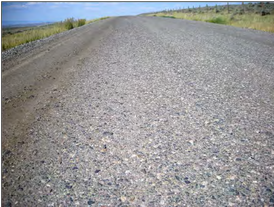
Figure 4.21 Road surface with some rutting on Johnson County's Schoonover Road, segment S1 with RAP and calcium chloride in August 2008, two months after RAP placement and one month after calcium chloride application.
