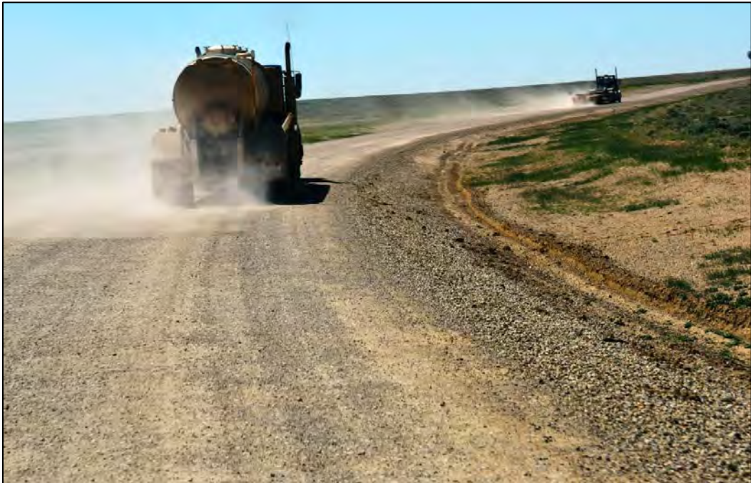
Figure 4.35 Dust from limestone crushed base before dust suppressant application on level, curved segment C on Sweetwater County's Crooks Gap Road in June 2011.
