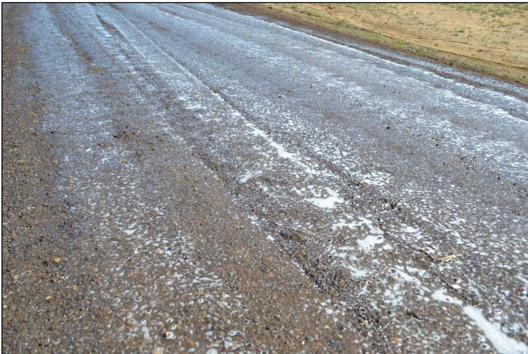
Figure 3.38 Recently applied magnesium chloride on the RAP and aggregate blend on Sweetwater County's Crooks Gap Road, July 2011.
