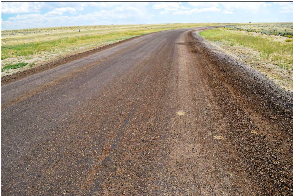
Figure 4.48 Road surface made from RAP blended with existing aggregate and treated with magnesium chloride on segment of Sweetwater County's Crooks Gap Road in August 2011, three weeks after application of dust suppressant.
