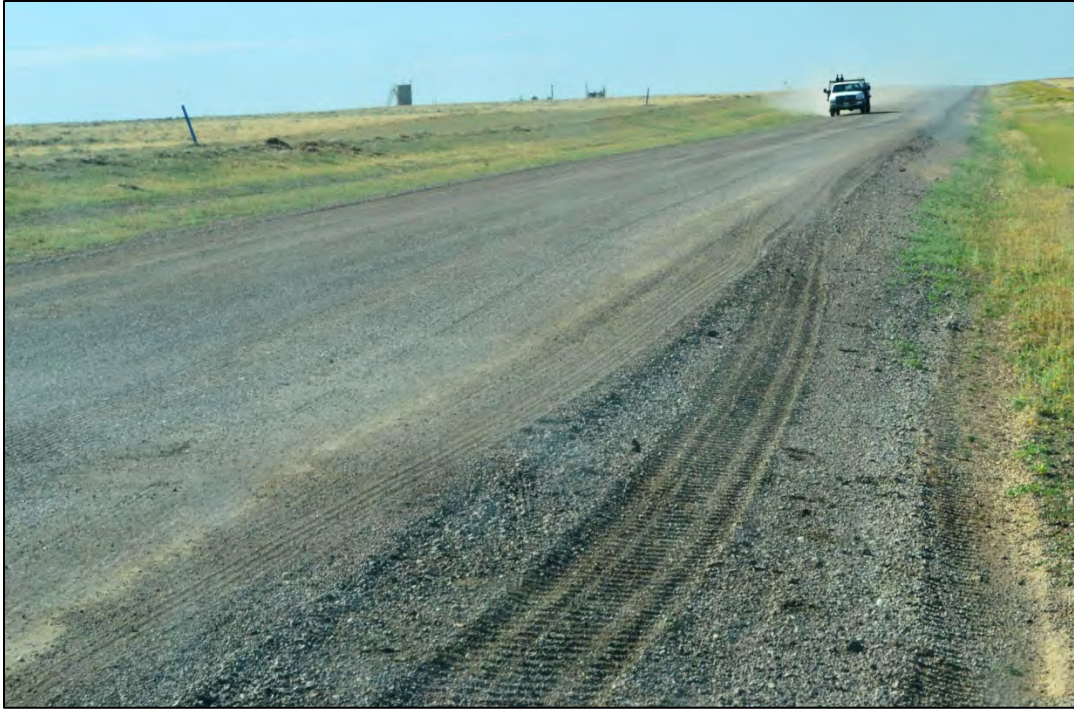
Figure 4.49 Road surface made from RAP blended with existing aggregate on segment P of Sweetwater County's Crooks Gap Road in August 2011.
