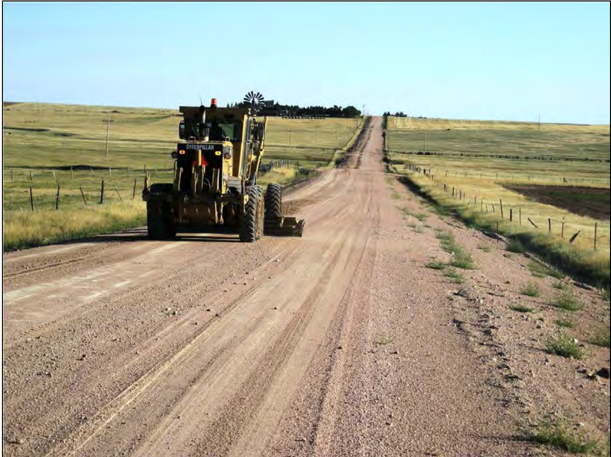
Figure 4.14 Re-working Laramie County’s Pry Road in August 2008, four months after initial application, to correct segregation with additional blending and spreading.
