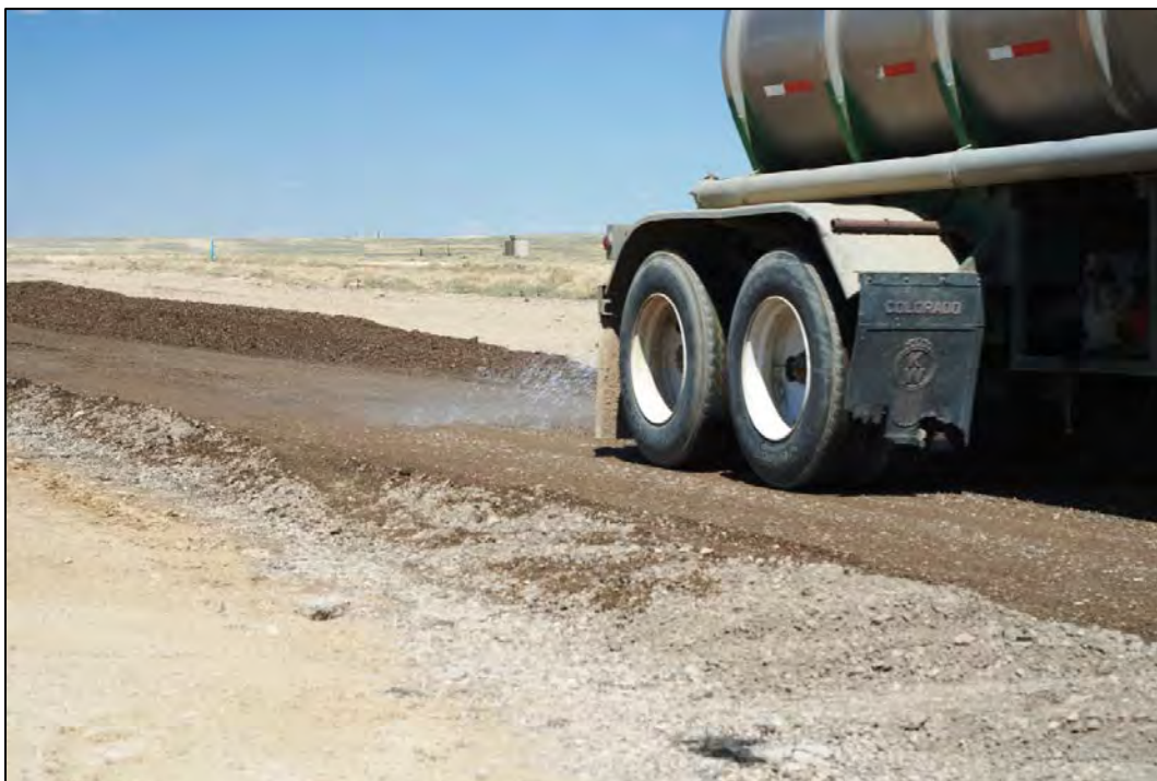
Figure 3.31 Applying water to the CTB and aggregate blend prior to final shaping and compaction on Sweetwater County’s Crooks Gap Road, August 2010.
