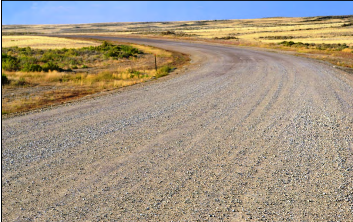
Figure 4.38 Broken up crust of limestone crushed base, foreground, and still intact crust, background, both treated with lignin and magnesium chloride on uphill, curved segment D of Sweetwater County’s Crooks Gap Road in September 2011, eight weeks after application of dust suppressant.
