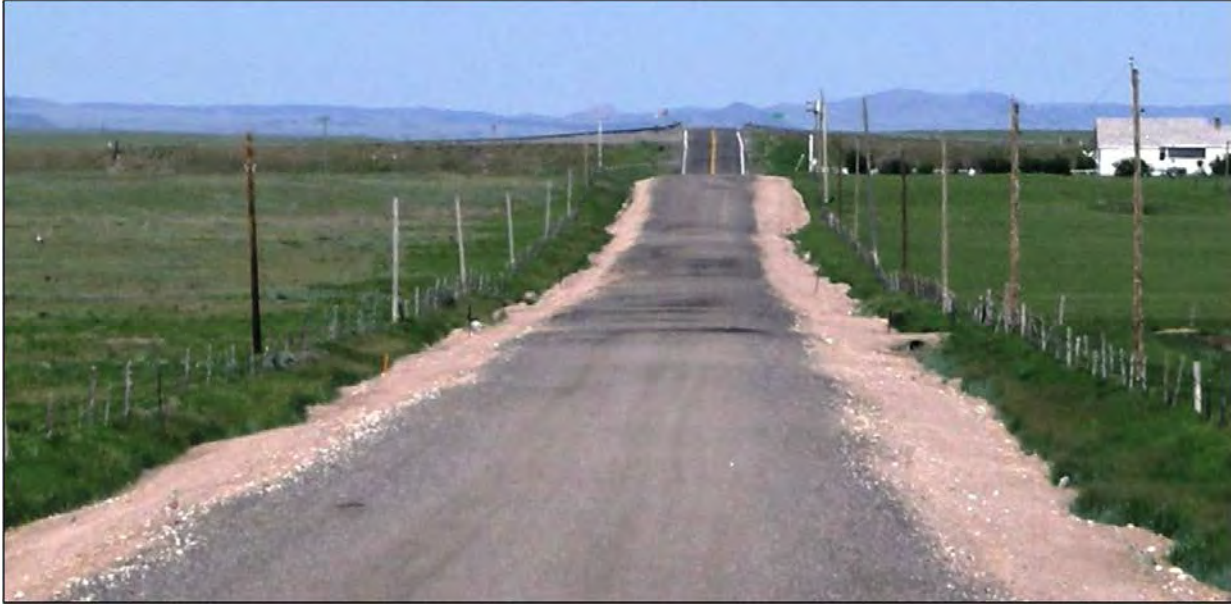
Figure 4.10 Segregation of RAP on Laramie County’s Atlas Road in June 2008, two months after initial RAP application.
