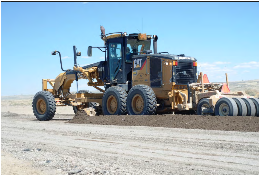
Figure 3.33 Final shaping and compaction of CTB and aggregate blend using a motor grader with pneumatic tire compactors mounted to its ripper hydraulics on Sweetwater County's Crooks Gap Road, August 2010.
