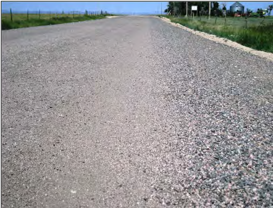
Figure 4.13 Well compacted, tight surface due to good blending on Laramie County's Atlas Road in June 2008, about two months after initial application.
