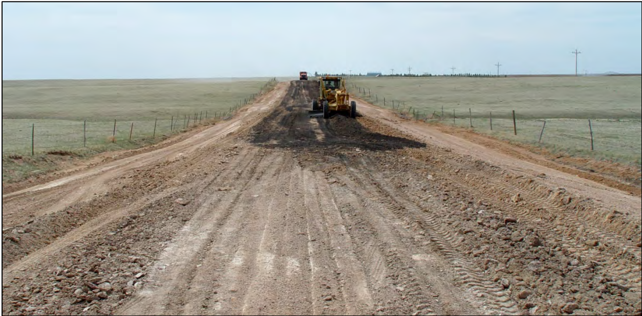
Figure 3.19 Blending and shaping RAP and existing, scarified aggregate on Laramie County's Atlas Road.
