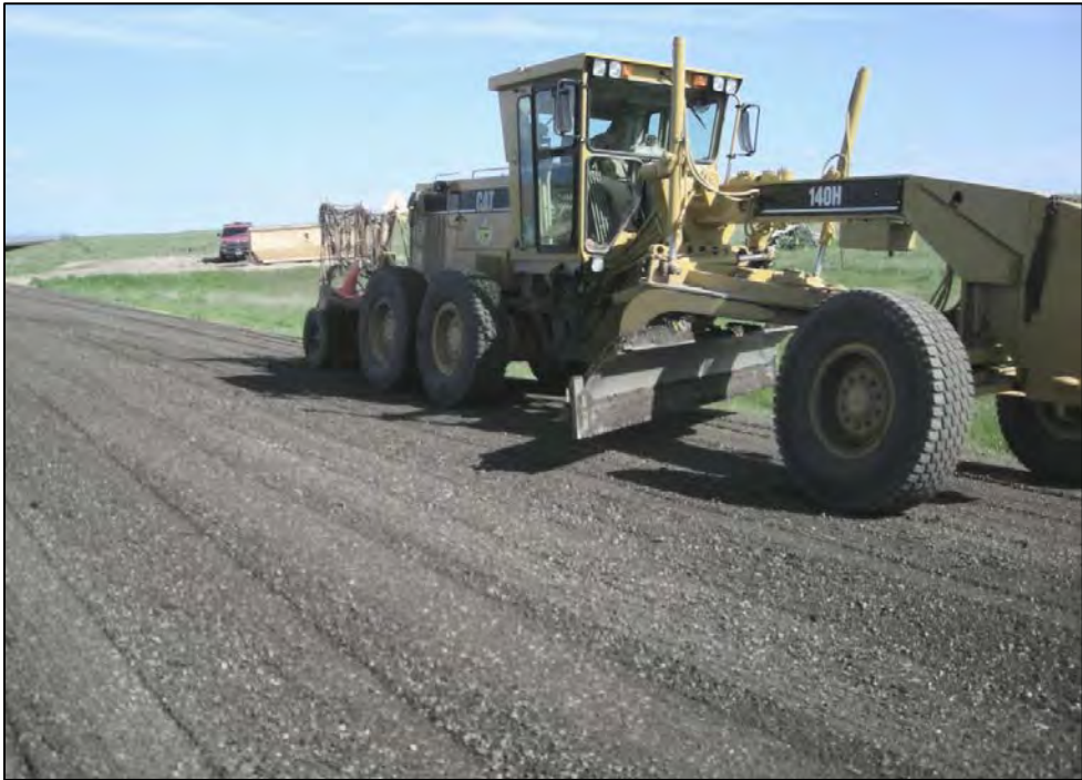
Figure 3.24 Compacting RAP and aggregate blend on Johnson County’s Schoonover Road with pneumatic tire compactors mounted on the motor grader’s ripper hydraulics, June 2008.
