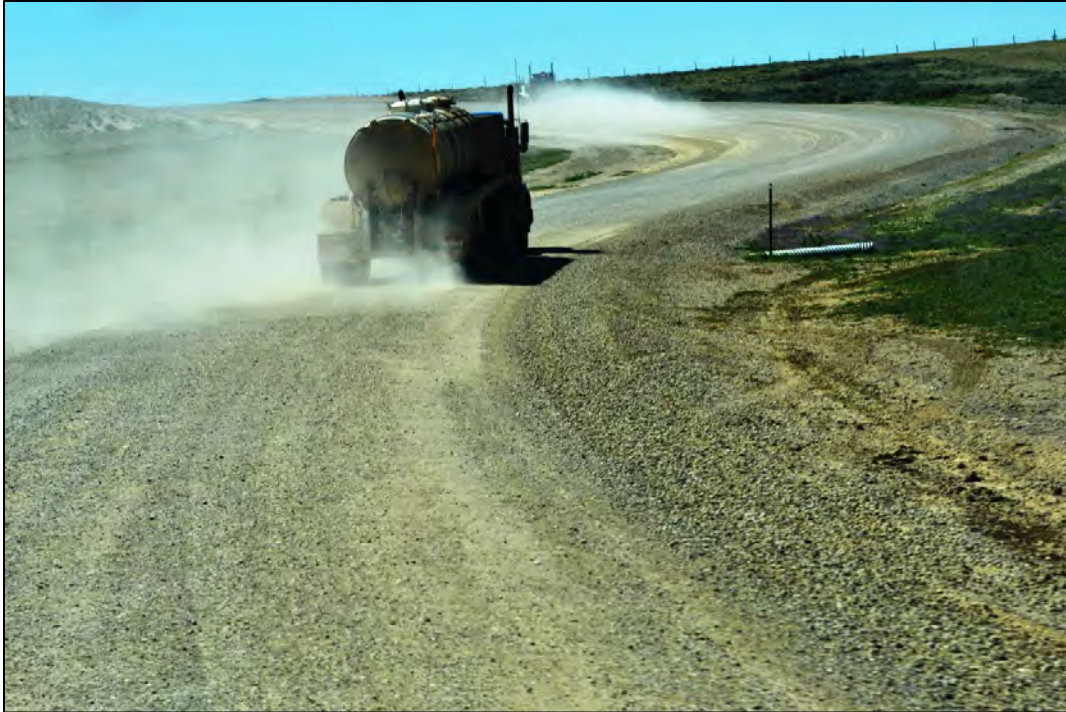
Figure 4.34 Dust from limestone crushed base before dust suppressant application on uphill, curved segment D of Sweetwater County's Crooks Gap Road in June 2011.
