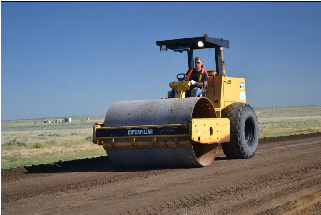
Figure 3.40 Compaction of the magnesium chloride-treated RAP and aggregate blend on Sweetwater County's Crooks Gap Road, July 2011.
