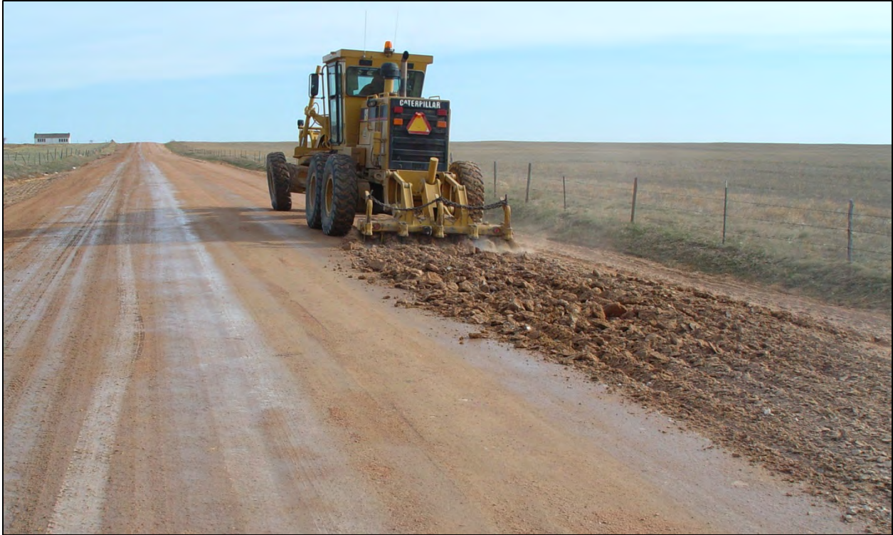
Figure 3.16 Scarifying Laramie County’s Atlas Road prior to placement and blending of RAP.
