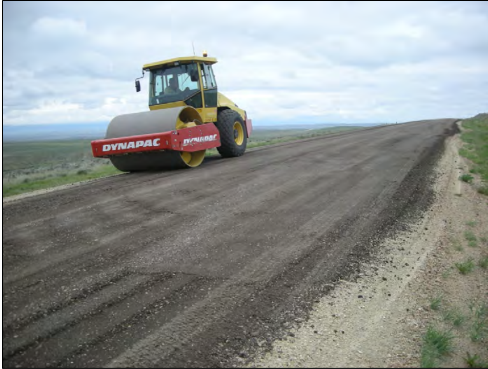
Figure 3.25 Final compaction of the RAP aggregate blend on County's Schoonover Road, June 2008.
