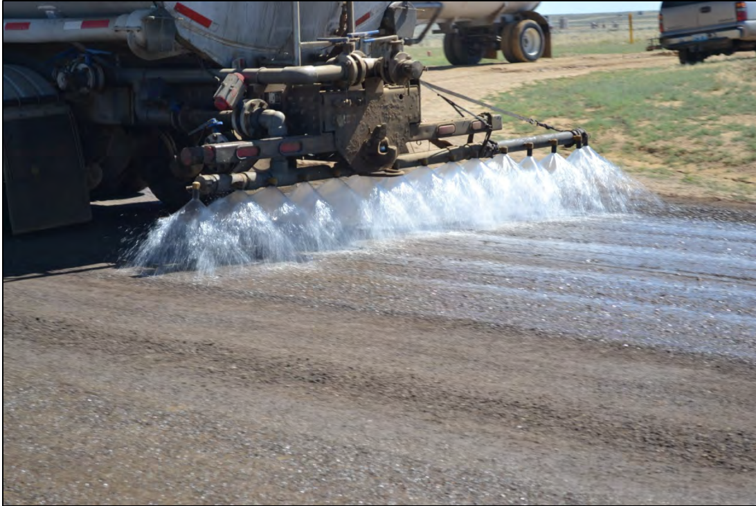
Figure 3.37 Applying dust suppressant brine to aggregate and RAP blend on Sweetwater County's Crooks Gap Road, July 2011.
