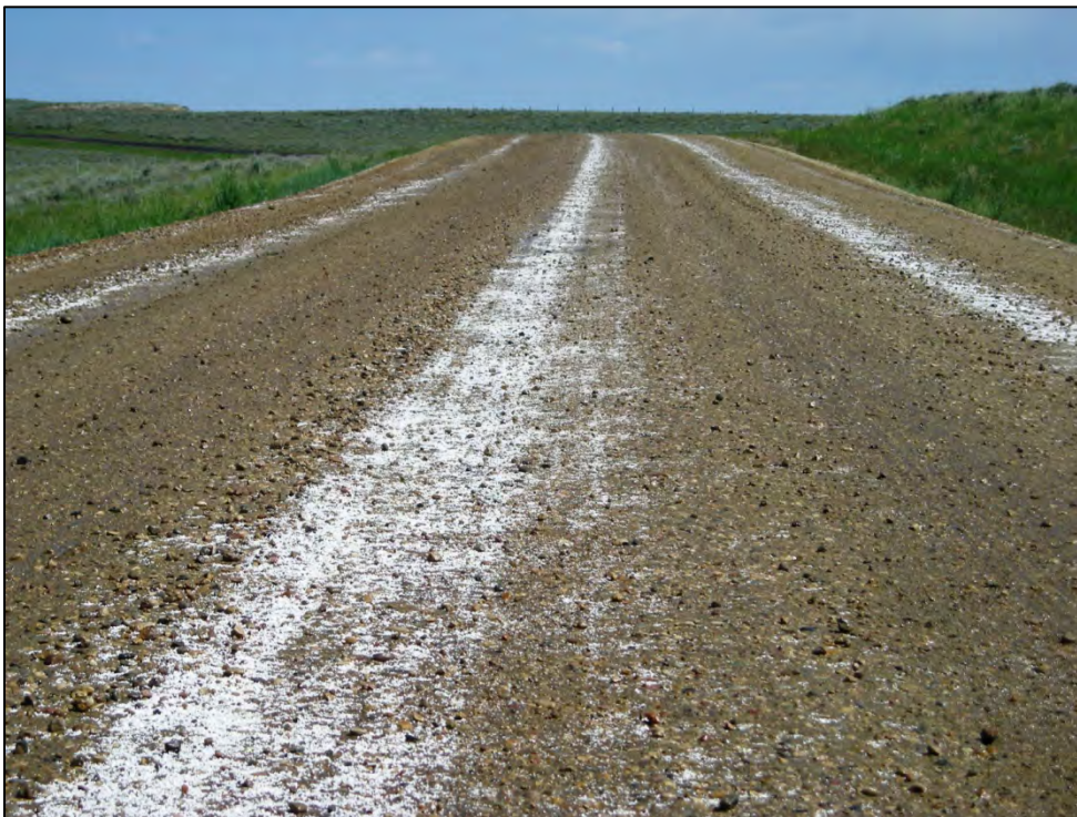
Figure 3.28 Calcium chloride flakes partially worked into the aggregate surface by traffic on Johnson County's Schoonover Road, June 2008.
