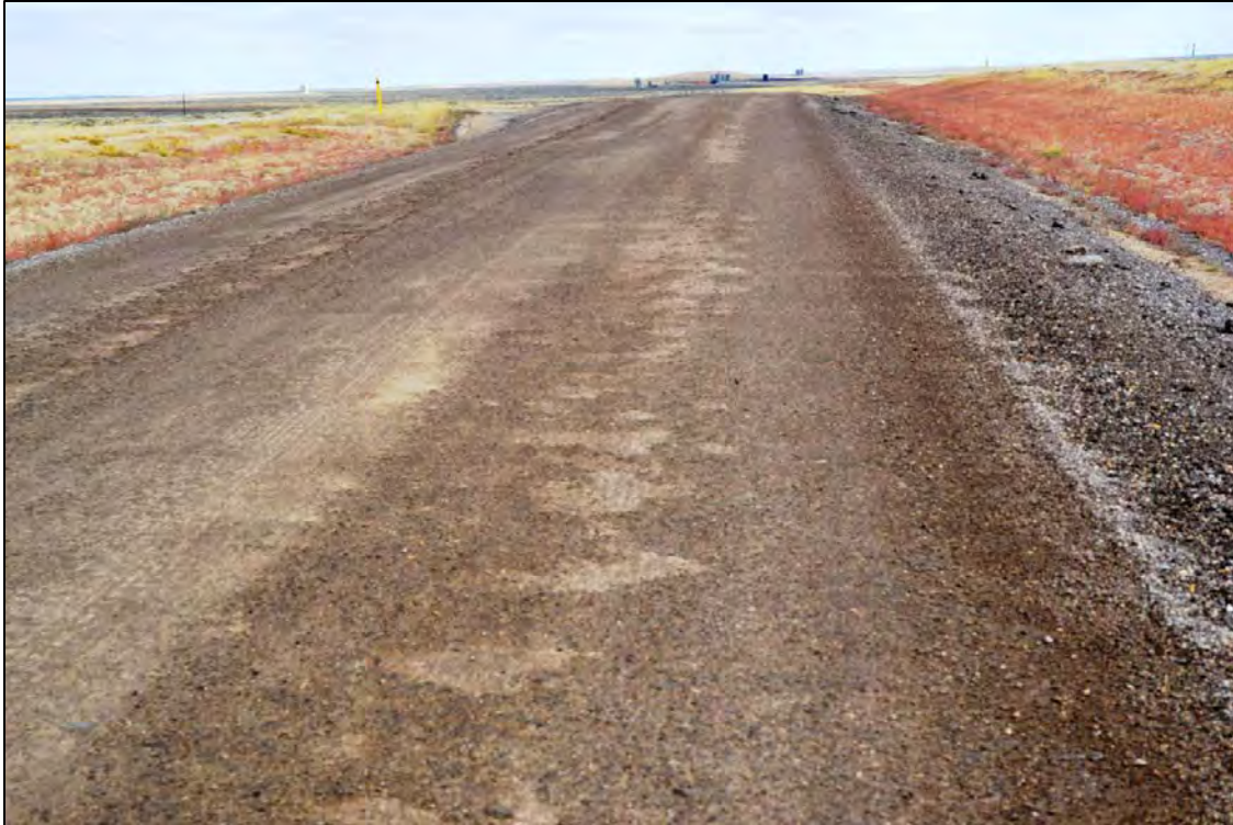
Figure 4.51 Road surface made with RAP blended with existing aggregate and treated with magnesium chloride and polymer on segment L of Sweetwater County's Crooks Gap Road in September 2011, eight weeks after application of dust suppressant.
