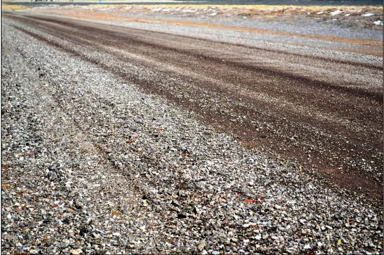
Figure 4.46 Road surface made from RAP blended with existing aggregate on segment Q of Sweetwater County's Crooks Gap Road in April 2011 without dust suppression agents.
