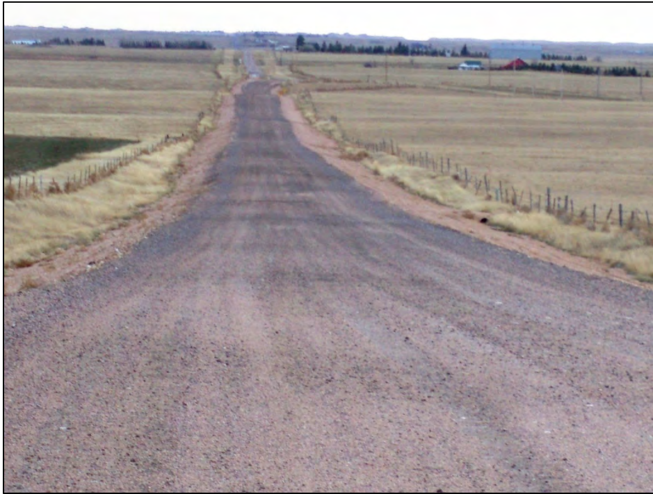
Figure 4.11 Segregation bands attributed to inadequate spreading of the windrows placed by the bottom-discharge haul trucks on Laramie County’s Pry Road in November 2008, six months after initial application.
