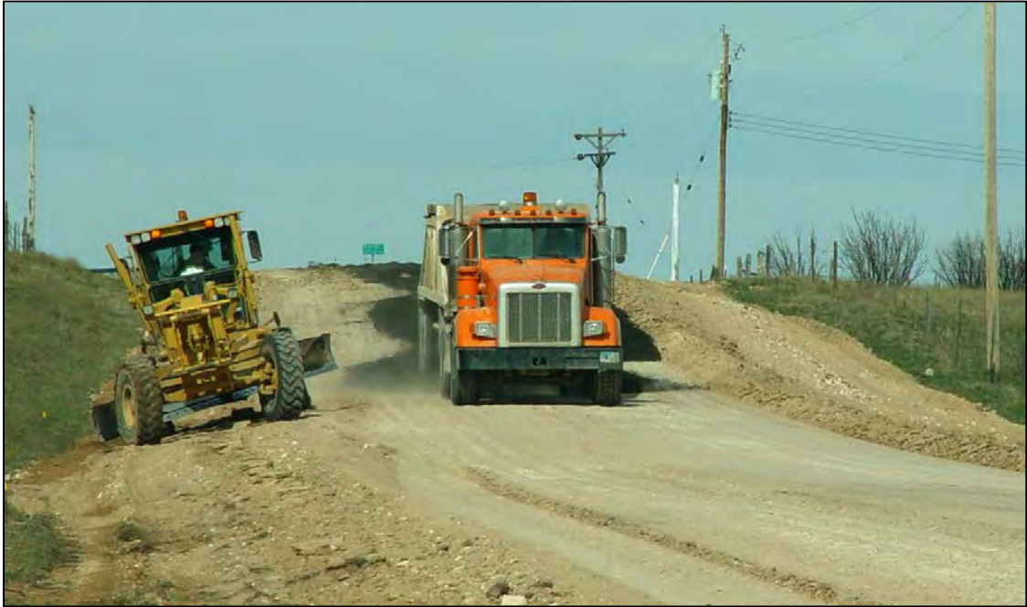
Figure 3.17 Placement of RAP windrow on Laramie County’s Atlas Road with bottom-discharge haul trucks.
