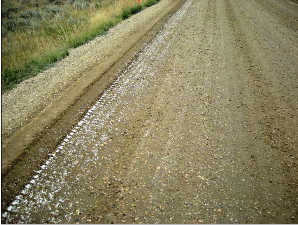
Figure 3.29 Calcium chloride flakes mostly worked into the aggregate surface by traffic on Johnson County’s Schoonover Road, June 2008.
