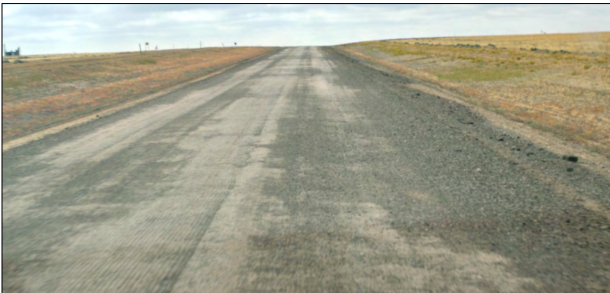
Figure 4.52 Road surface made with RAP blended with existing aggregate on segment P of Sweetwater County's Crooks Gap Road in September 2011.
