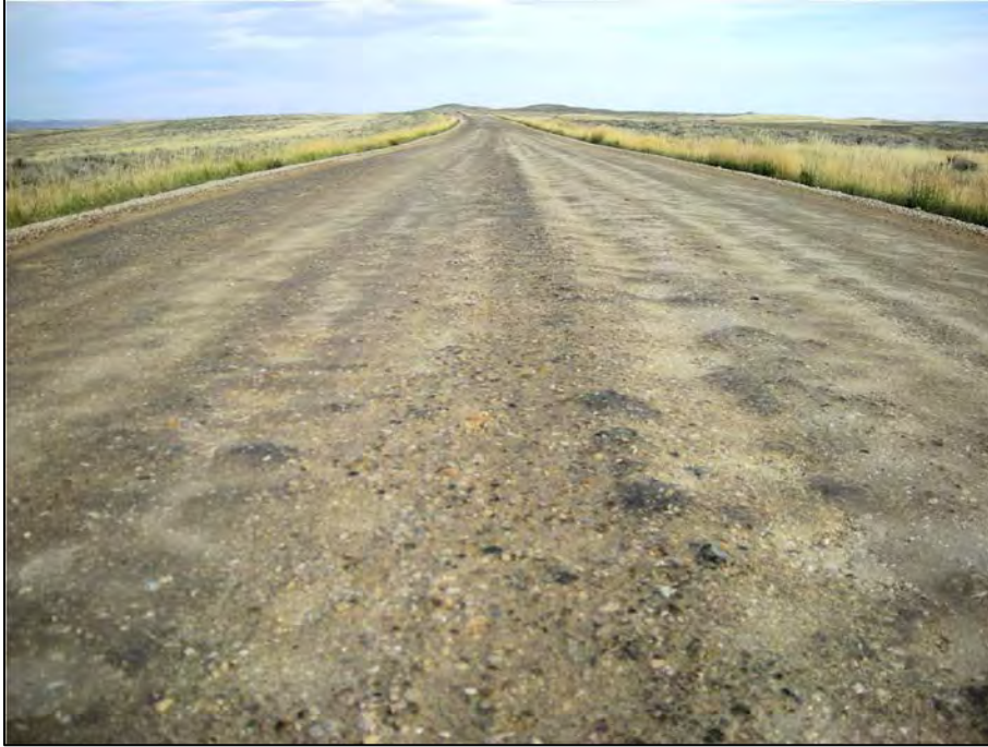
Figure 4.24 Road surface on Johnson County's Schoonover Road, segment S1 with RAP and calcium chloride in October 2008, four months after RAP placement and three months after calcium chloride application.
