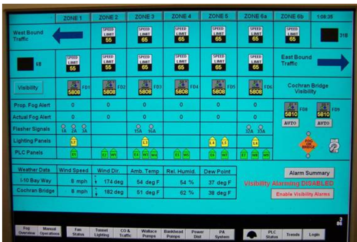
Figure AL-1. Screen Shot of Low Visibility Warning System.
