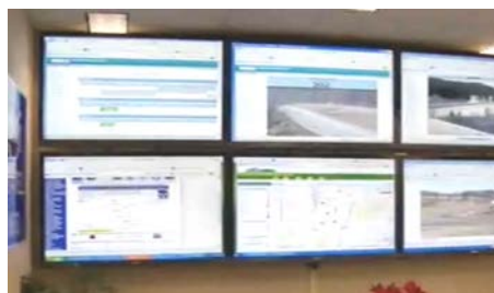
Figure VT-1. Traffic operations center.
