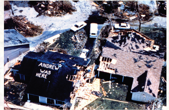
Hurricane Andrew damage
