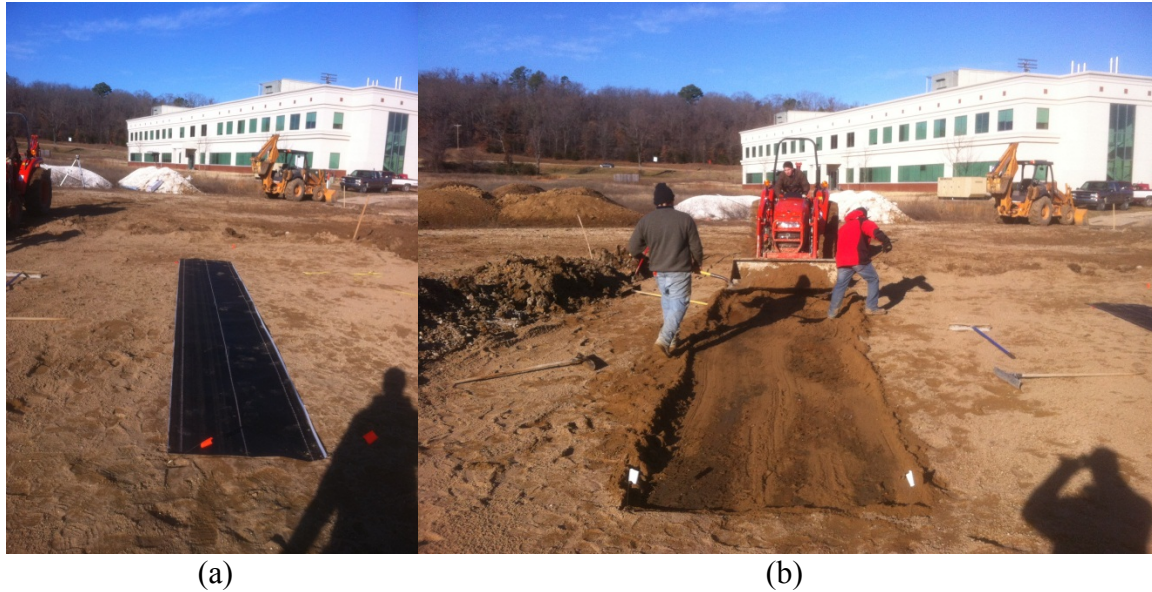
Figure 3.14. (a) Geosynthetic membrane in place on sand blanket of Pad 1. (b) Excavating the sand blanket prior to placement of gravel pad in Pad 1.
