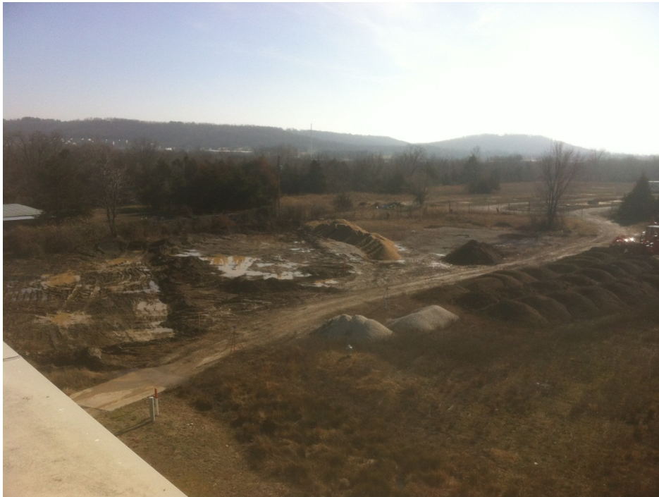
Figure 3.12. Project under construction showing stockpile locations, spoil heaps, and rough grading underway.
