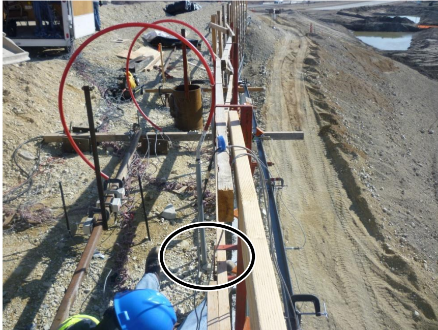
Figure 5.31: Shape Array casing in line with TP4 separated from wall by a couple inches.
