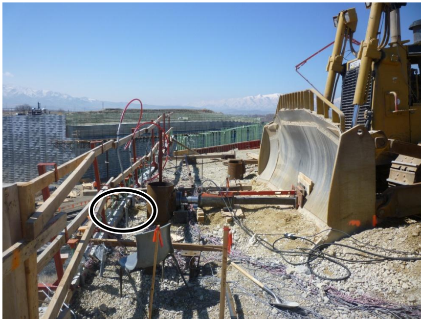
Figure 5.32: Shape Array casing in line with TP5 separated from wall by a couple inches.
