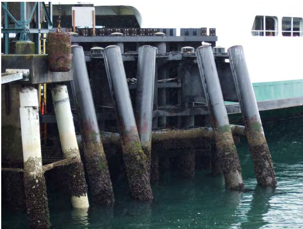
Figure 6: Posterior of WSF wingwall at Seattle terminal
