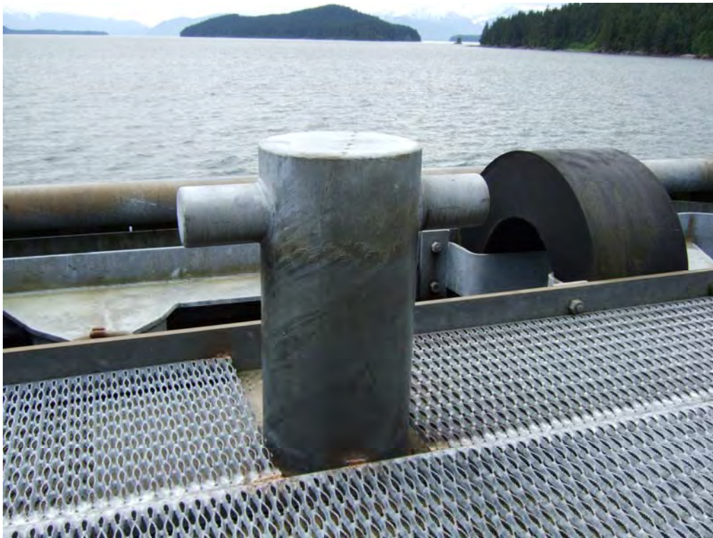
Figure 5: Typical Bollard at AMH Auke Bay Terminal; Note “doughnut” fender behind bollard
