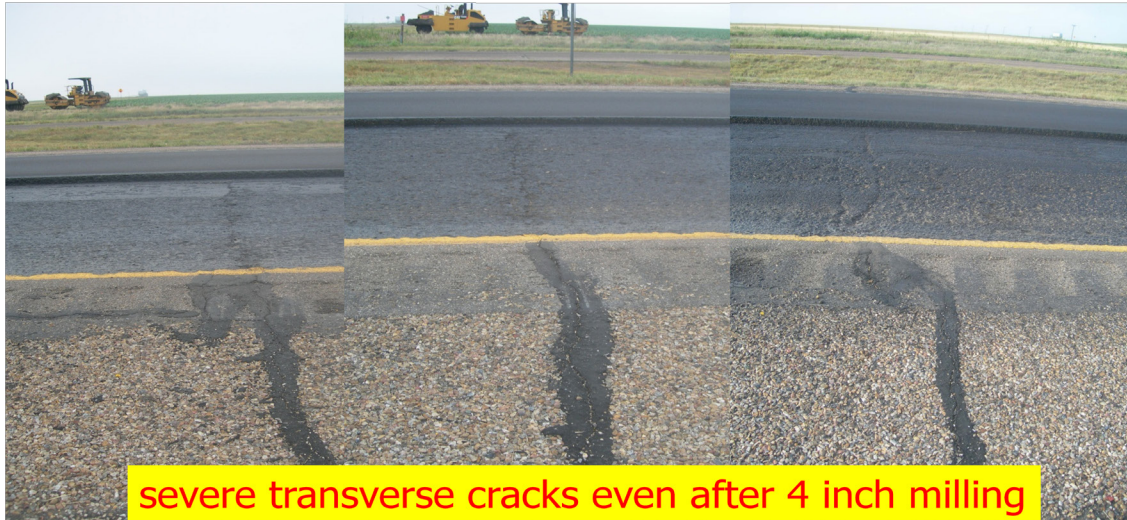
Figure B3. Existing Pavement Conditions of IH40 after Milling.
