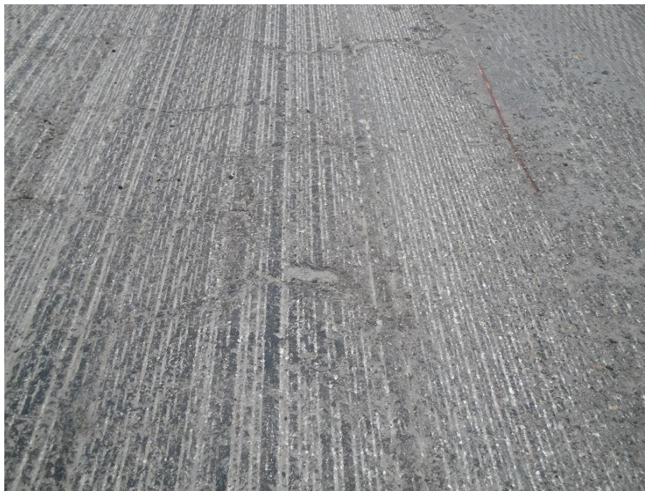
Figure 5. Observed Cracking after 3 inch Milling on SH359.
