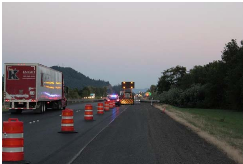
Figure 3.18: OSP Parked at the End of Taper for I-5 Case Study Project
