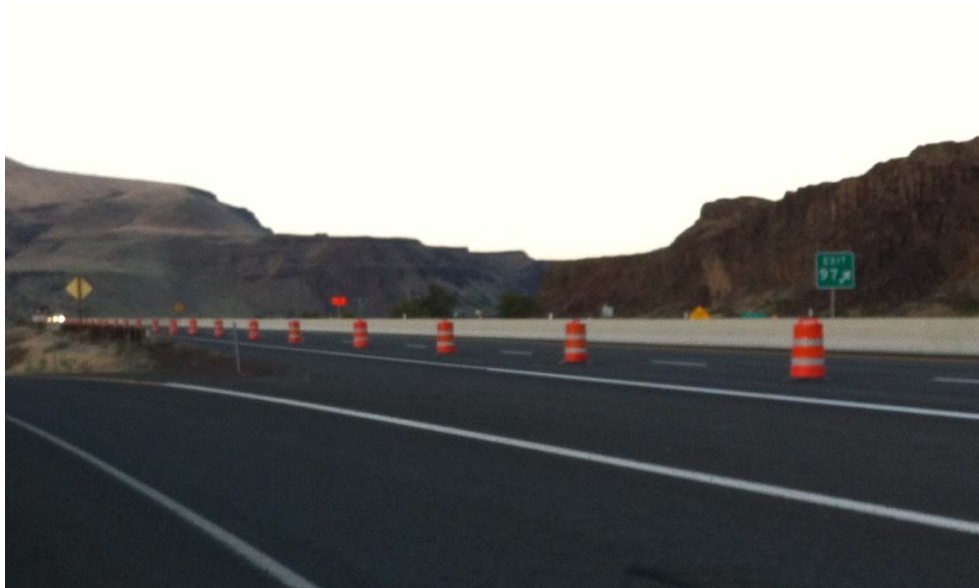
Figure 2.3: Plastic Drums on Roadway
