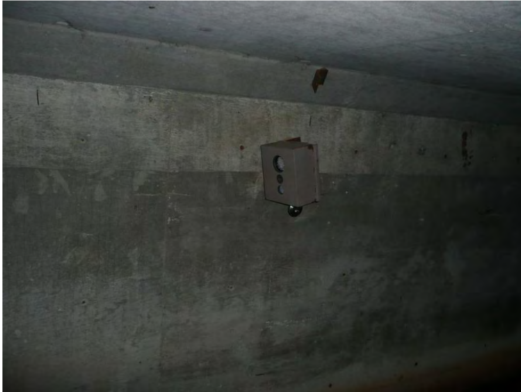
Figure 3.3. Remote camera deployed on culvert wall in a locked, metal security box. (Photo: R. Long/WTI)
