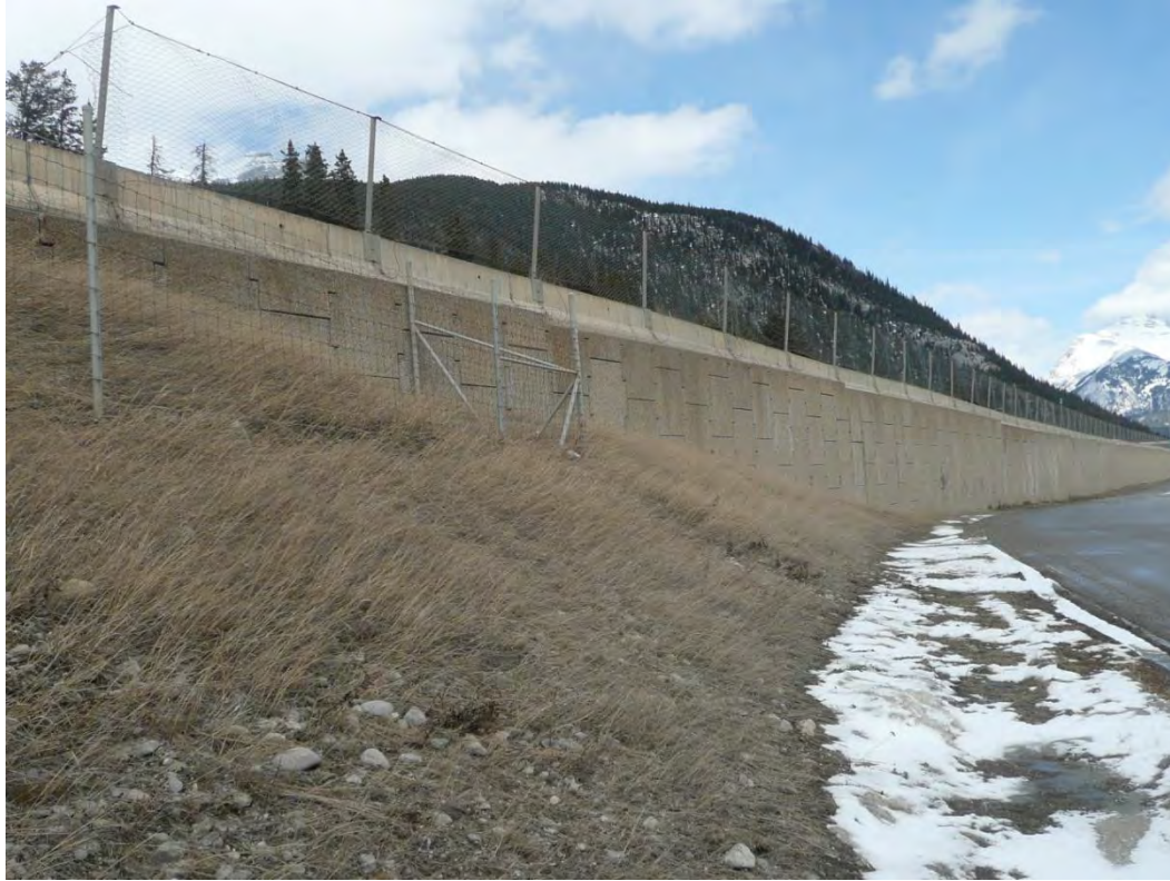
Exhibit 5. Mechanically stabilized earth (MSE) retaining wall along the Trans-Canada Highway in Banff National Park, Alberta. (copyright: Tony Clevenger)
