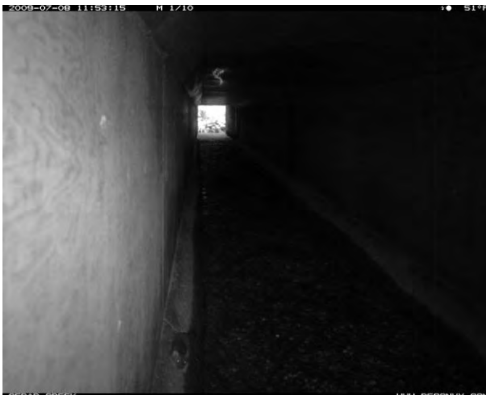
A weasel passing through the Cedar Creek Culvert. (Photo: WTI)
