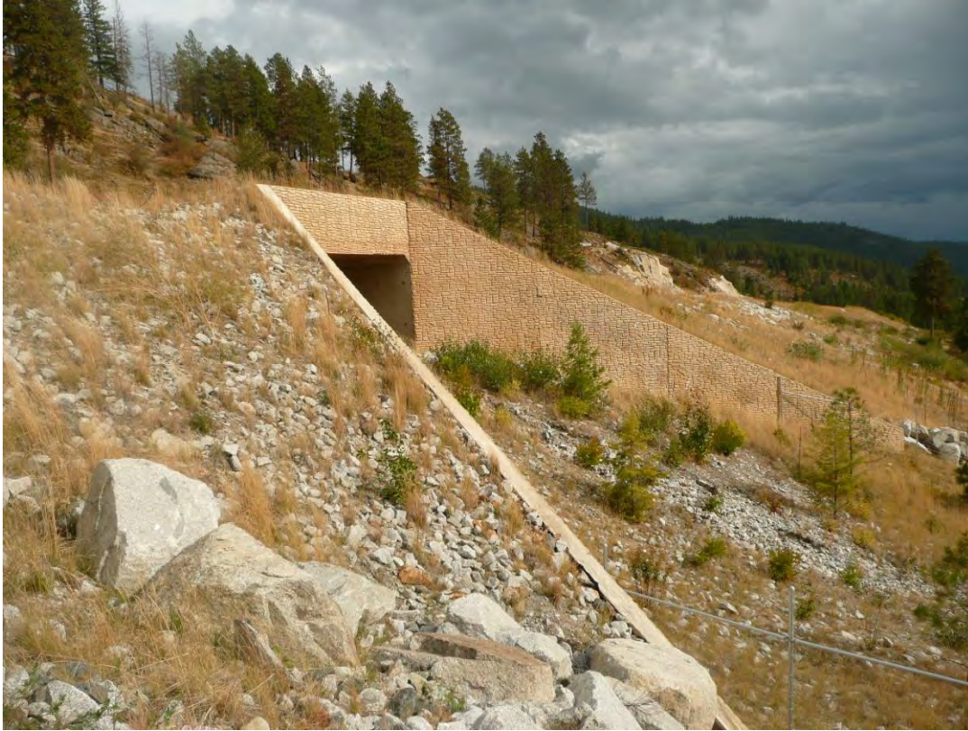
Exhibit 11. Retaining wall at wildlife underpass on US 95 near Bonners Ferry, Idaho. (copyright: Tony Clevenger).
