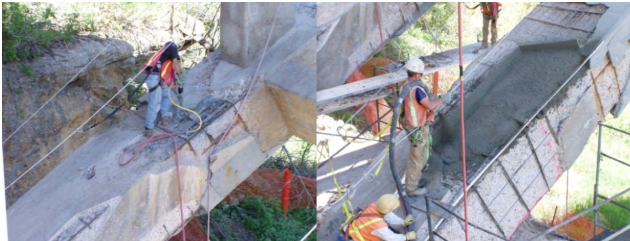
Figure 2.9 Removal of loose concrete using 6.8 kg (15 lbs.) jackhammer and restoring the cross section with shotcrete (Mohseni, CDOT)
