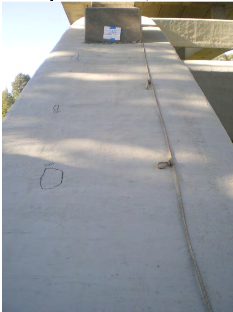
Figure A6. Bay 2NE, 3 Voids
