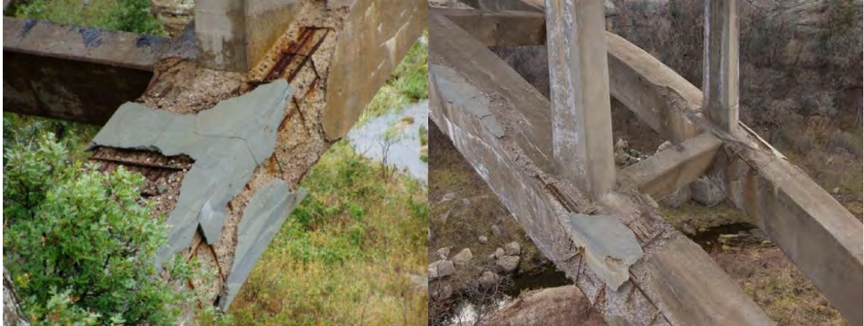
Figure 2.8 Concrete spalling on arch section prior to repair (Mohseni, CDOT)
