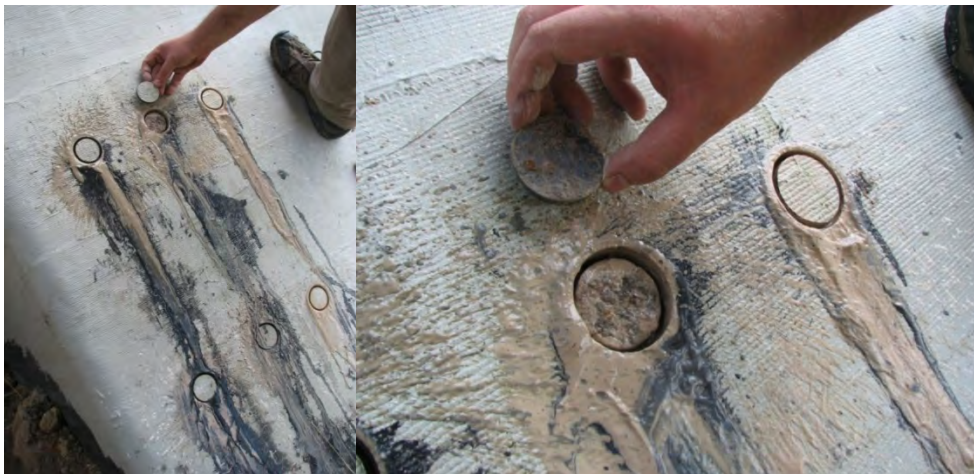
Figure 3.6 The core drilling location that failed due to torsional stresses during the core drilling process, bay 1NW
