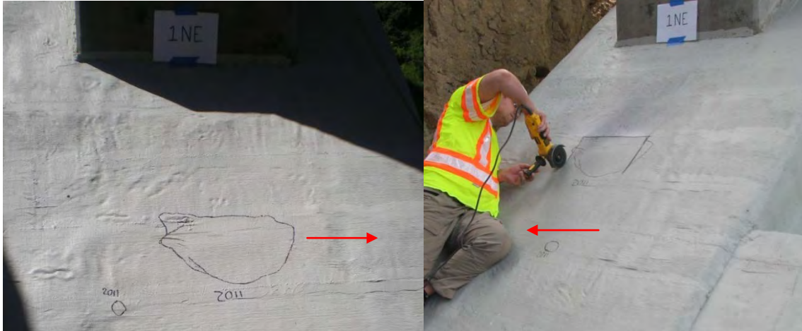
Figure 3.20 Void in CFRP with transverse crack identified with red arrows and Cutting the perimeter of the void in the CFRP
