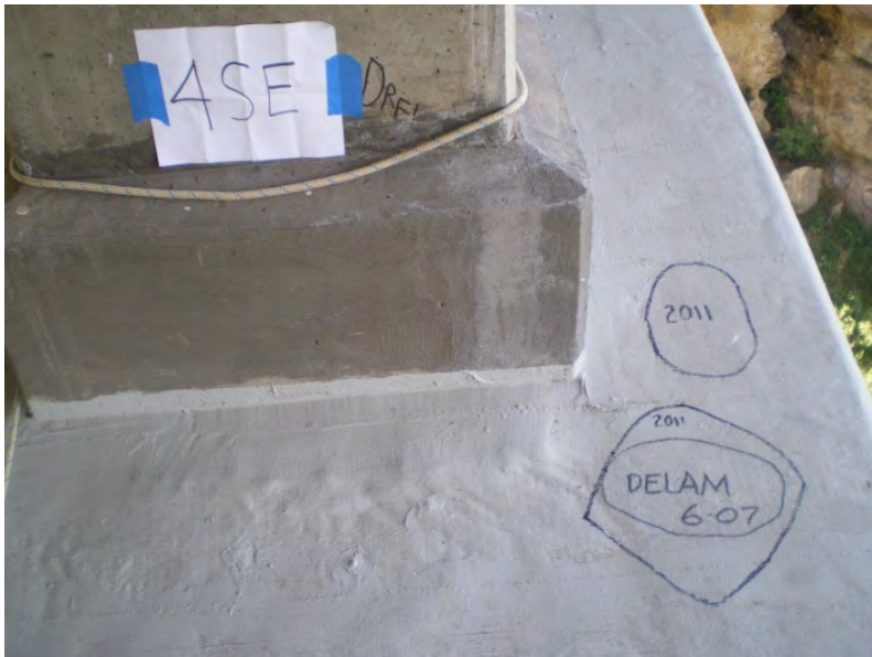
Figure 2.15 Enclosed in permanent marker are identified areas of debonded areas between the FRP and the substrate from 2011 and June, 2007. Notice in this more protected bay of the structure the markings from 2007 are more clearly visible.
