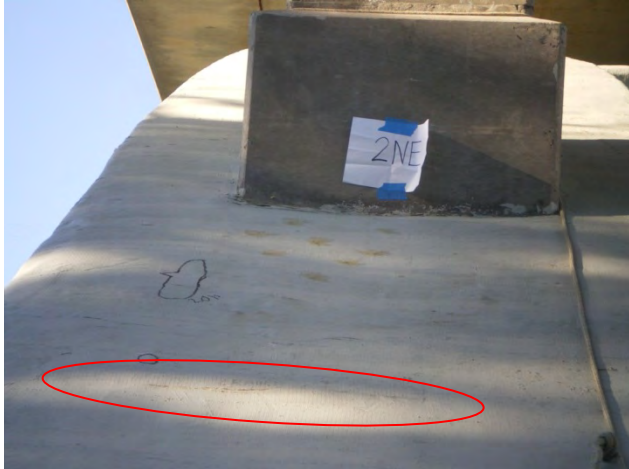
Figure 2.16 Crack identified in 2007
