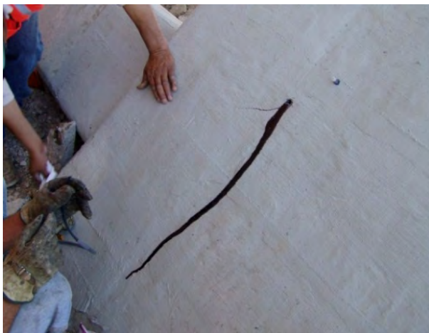
Figure 2.12 Void injected with resin during 2003 renovation (Mohseni, CDOT)
