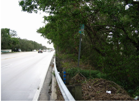
(a) No loading area, no sidewalk, and with physical barriers.
