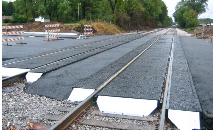
Figure 3-11: Full-Depth Heavy-Duty Rubber System (Source: OMNI Grade Crossing, 2012c)
