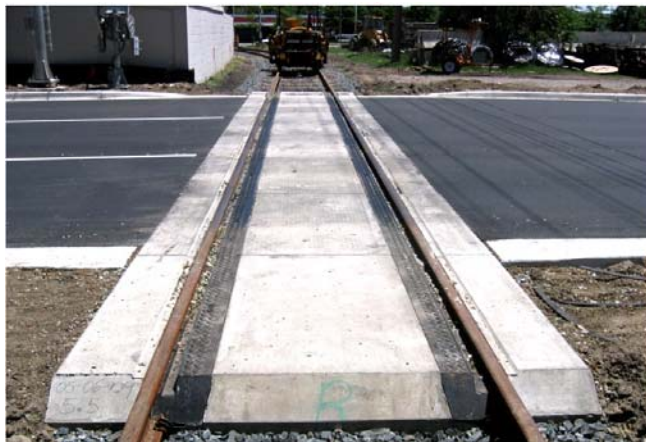
Figure 3-4: TraCast Crossing System (Source: OMNI Grade Crossing, 2012b)
