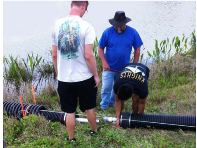
Researchers install a pipe-in-pipe filtration apparatus next to a pond on the UCF campus.
