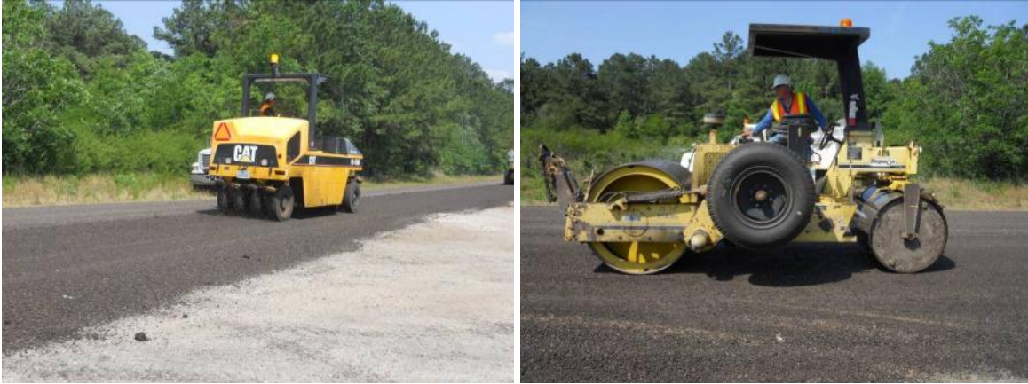
Step 4: Compacting the mix with pneumatic compactor and finishing with steel wheel compactor.
