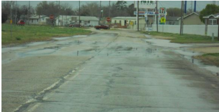
Figure 4-3. Depressions on the Pavement Surface Causing Water Collection.
