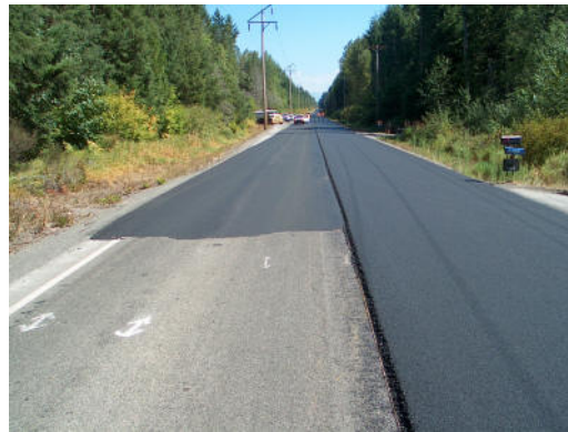
Figure 2-3. Photo Showing the Existing Pavement (Left, Front), a Leveling Course (Left Rear), and the Final Surface Course (Right) (after WSDOT 2011).
