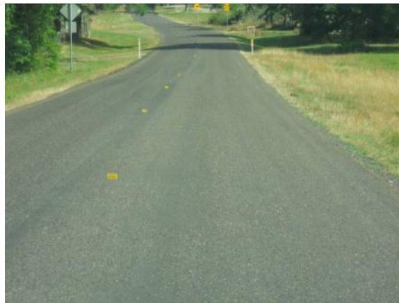
Step 5: Installing temporary reflectors, removing the traffic controls and opening for traffic.
