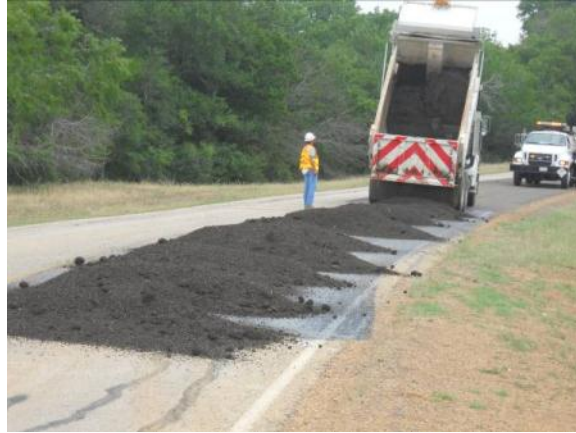
Step 5: Laying down the patching mix with dump truck in multiple piles over the tacked areas.
