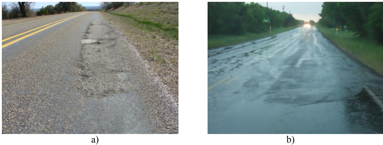
Figure 4-6. Patch Deterioration in the Form of a) Improper Mix Design and Compaction and b) Corrugation and Roughness due to Insufficient Compaction.
