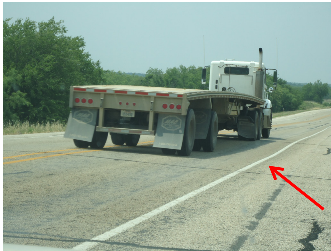
Figure 4-1. Example of Pavement Depression.
