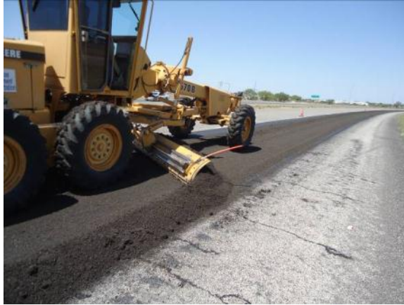
Step 3: Blading the mix along the full lane in several passes until it becomes flush with the existing cross slope.
