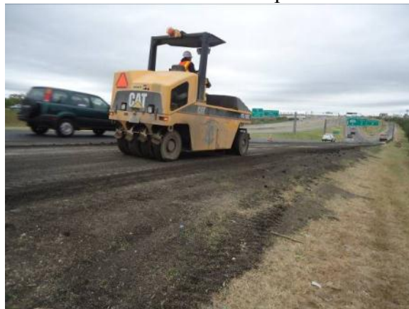
Step 6: Pneumatic compacting of the 0.5-inch patching layer. Better compaction is achieved with thin lifts.
