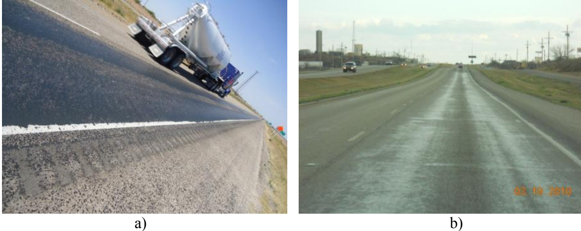
Figure 4-5. Asphalt Bleeding a) across the Travel Lane and b) in the Wheel Path Reducing the Skid Resistance Particularly in Warm Temperatures.
