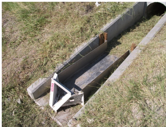
Figure 9. H-Flume at the Influent Location to Measure Flow.
