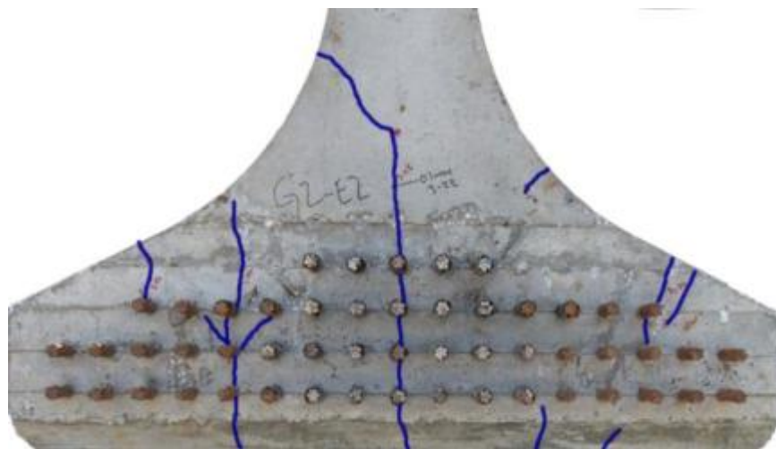
Figure 13–Flange splitting in experimental girder.
