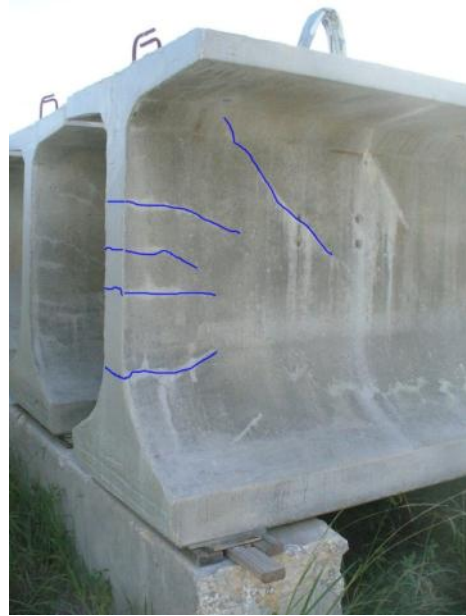
Figure 1–Web splitting cracks (enhanced in blue)
