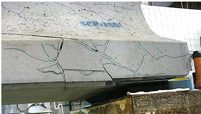
Figure 73–Bottom flange cracking at SL bearing.
