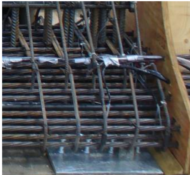
Figure 42–Wire harness and plywood bulkhead
