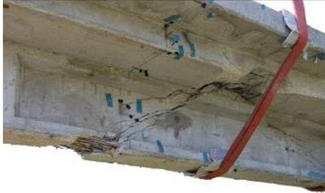
Figure 16–X7 punching failure bottom view
