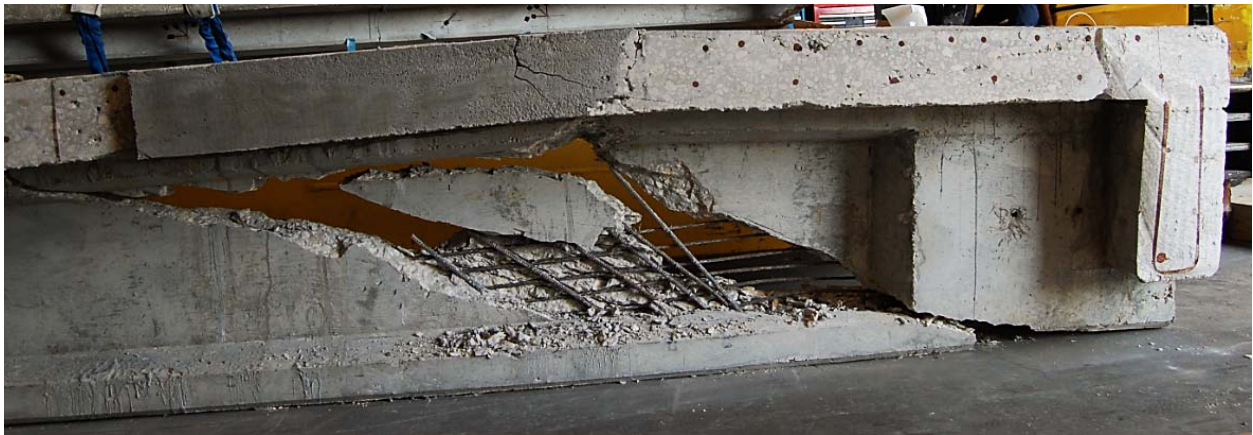
Figure 30-I2A transverse reinforcement-arch failure
