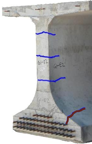
Figure 23–Web splitting (blue) and flange splitting (brown) cracks
