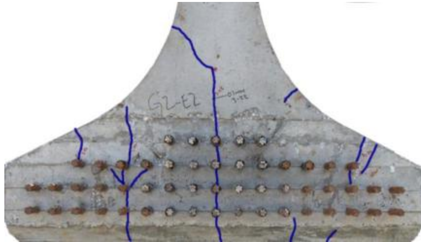
Figure 53–Flange splitting in experimental girder
