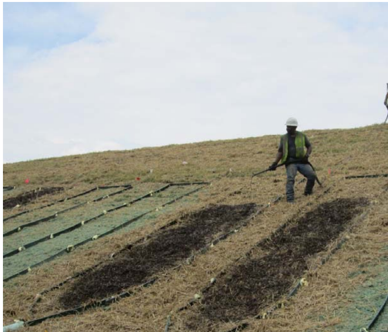
Figure 5: Straw cover and excessively applied tackifier at Site 5, Holly Springs, NC.
