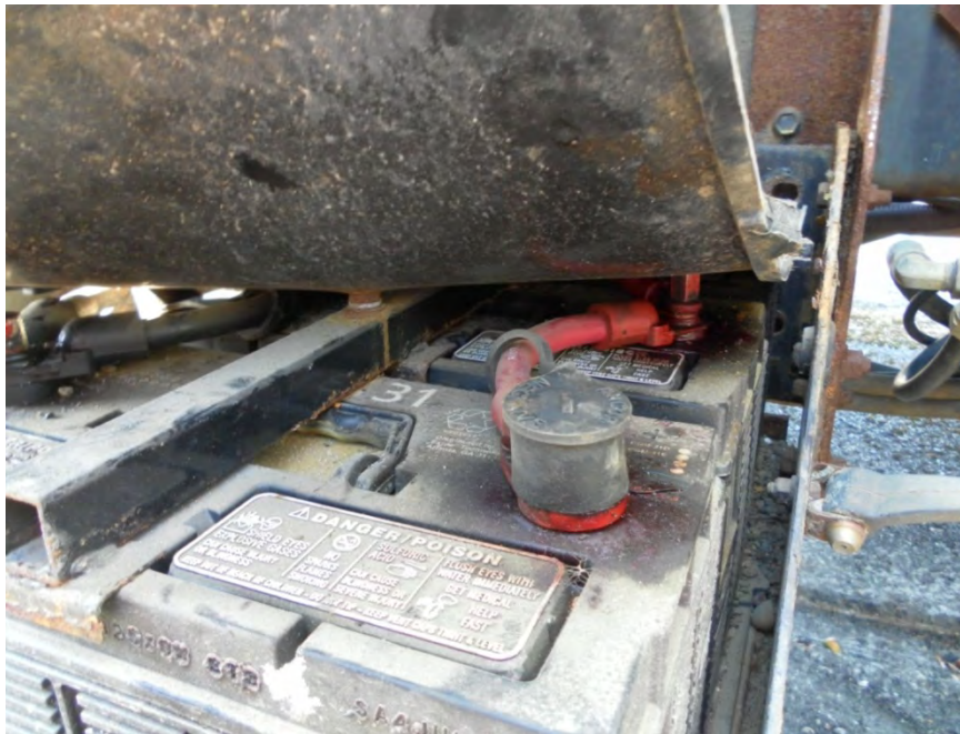
Figure 41. Rubber caps on battery terminals used to mitigate effects of corrosion.
