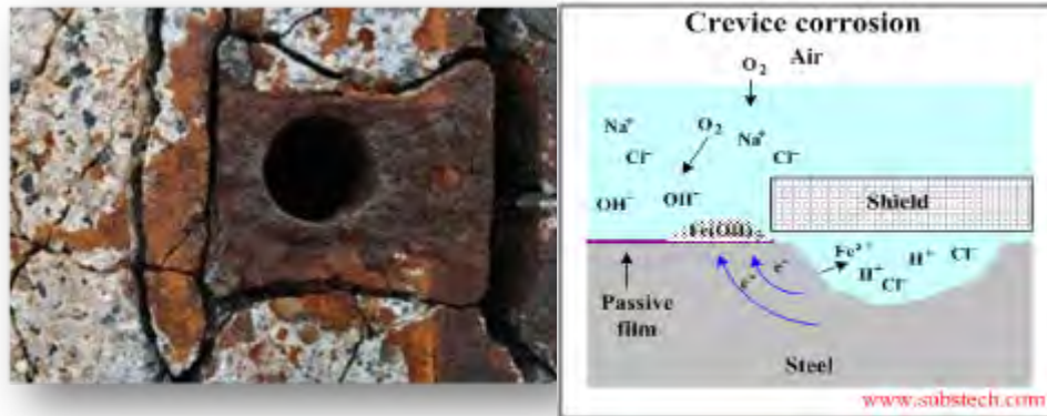
Figure 1 Crevice corrosion (Kopeliovich, 2009)
