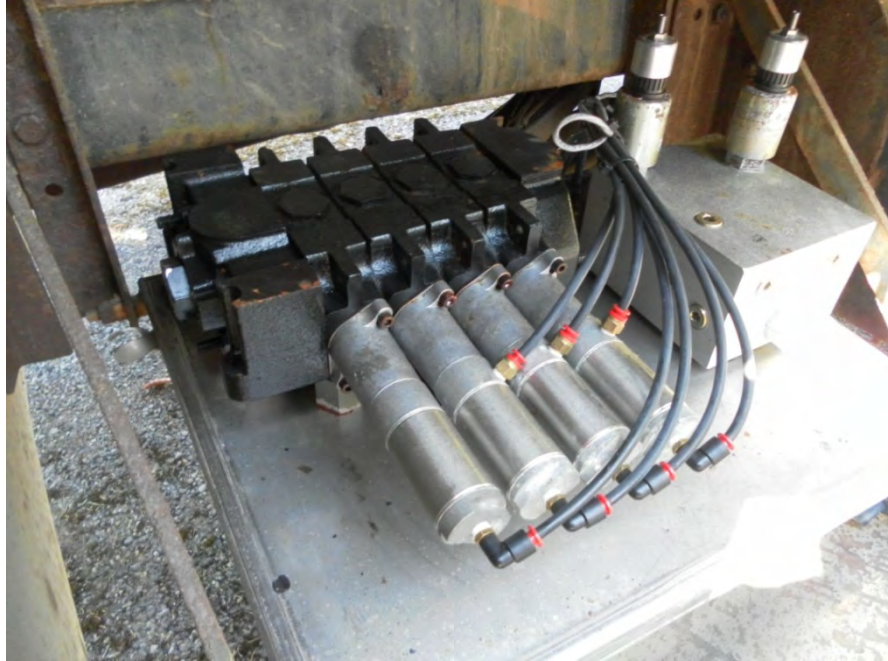
Figure 38. Hydraulic components showing little to no corrosion due to sealed protective cover.
