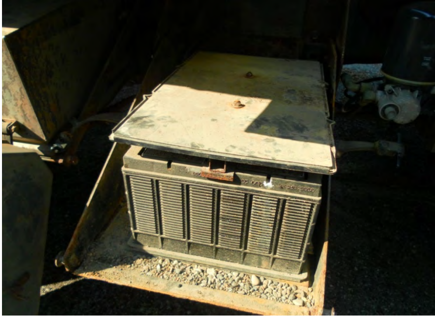
Figure 40. Modified protective cover for battery to reduce harmful effects of corrosion.
