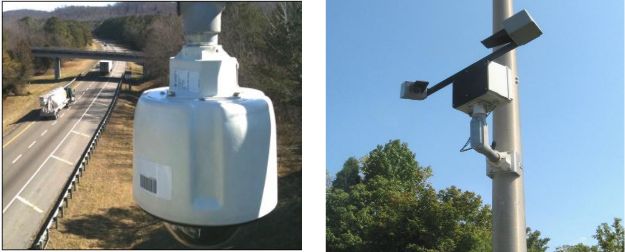
Figure 12 Installed Visibility Sensor and CCTV camera along I-75
