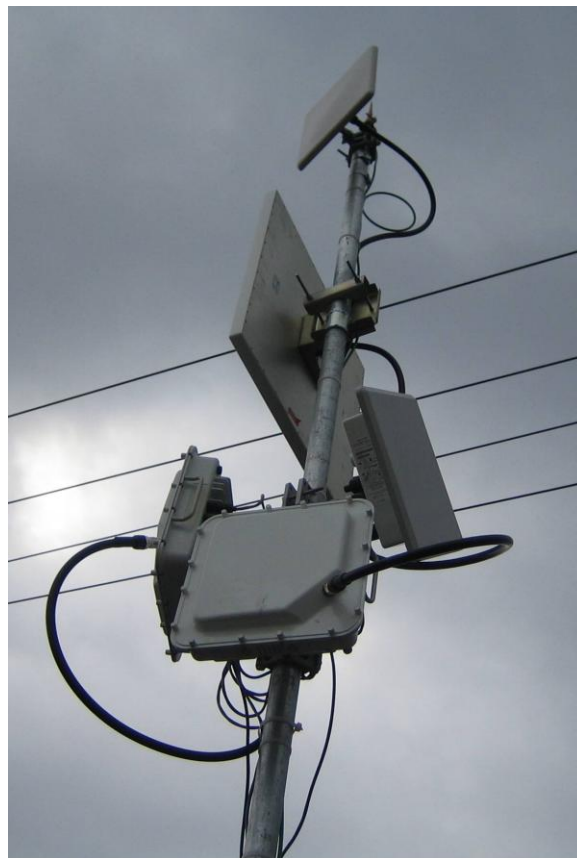
Figure 7-Visibility Sensors Installed by Caltrans
