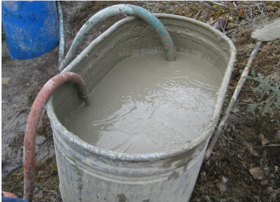
Figure D-2. Cement-bentonite grout during the back-filling process. (Photograph by M. Darrow, Sept 2012)
