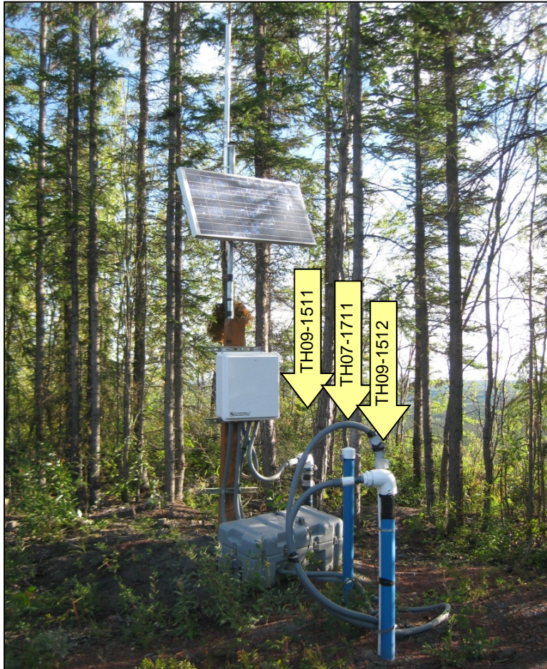
Figure 4. Relative locations of the measured casings at Rich113. Vertical arrows are labeled with the test hole identifiers. The edge of the bluff overlooking the Copper River is immediately beyond the spruce trees behind the installations, and the Richardson Highway is behind the photographer. (Photograph by M. Darrow)
