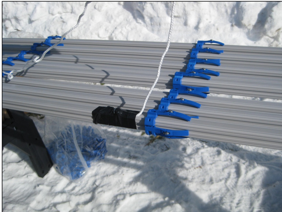
Figure A-8. Attaching the safety line to the lowest module. (Photograph by M. Darrow, March 2010)
