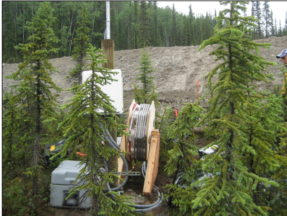
Figure C-11. Installation of SAA device, showing shipping reel position relative to embankment and ADAS. (Photograph by M. Darrow, July 2012)
