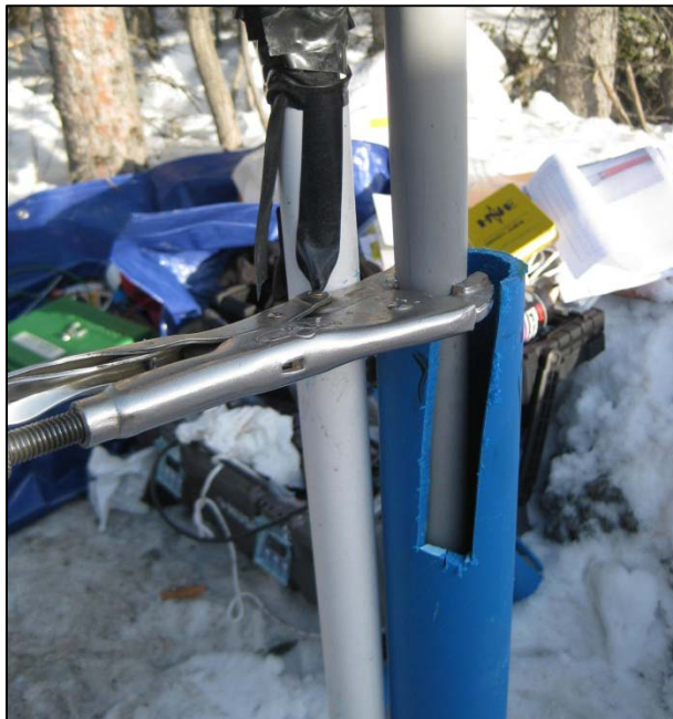
Figure A-13. Installing inner 1.05-in. PVC into guide casing for SAA device. Slot cut into the guide casing was to allow tightening of the hose clamp at the top of the PVC casing (see Figure A-14). White 1-in. PVC to the left was for a thermistor string. (Photograph by M. Darrow, March 2010)
