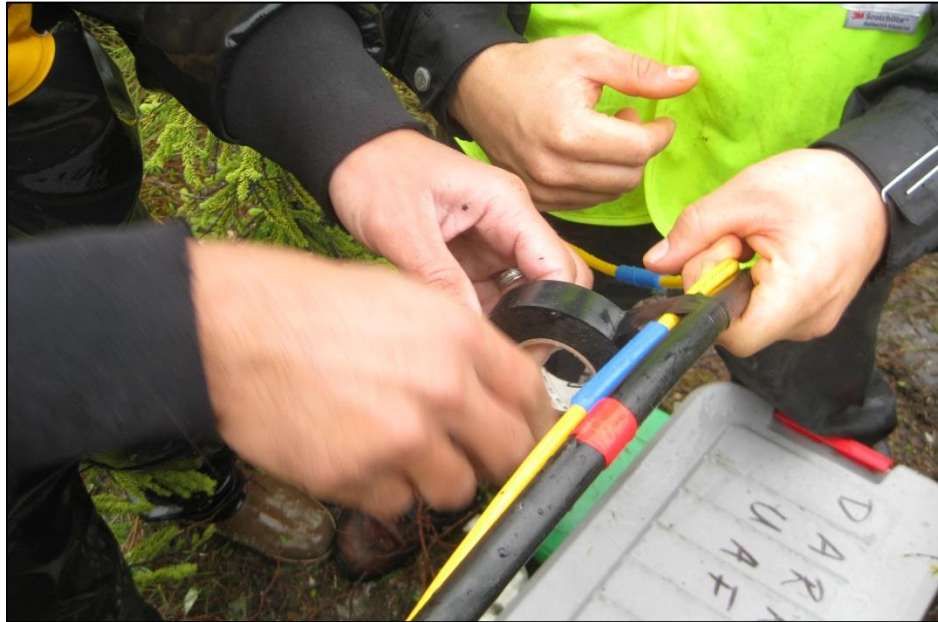
Figure C-5. Wrapping BeadedStream temperature acquisition cable (TAC) to thermistor cable for installation. (Photograph by M. Darrow, July 2012)
