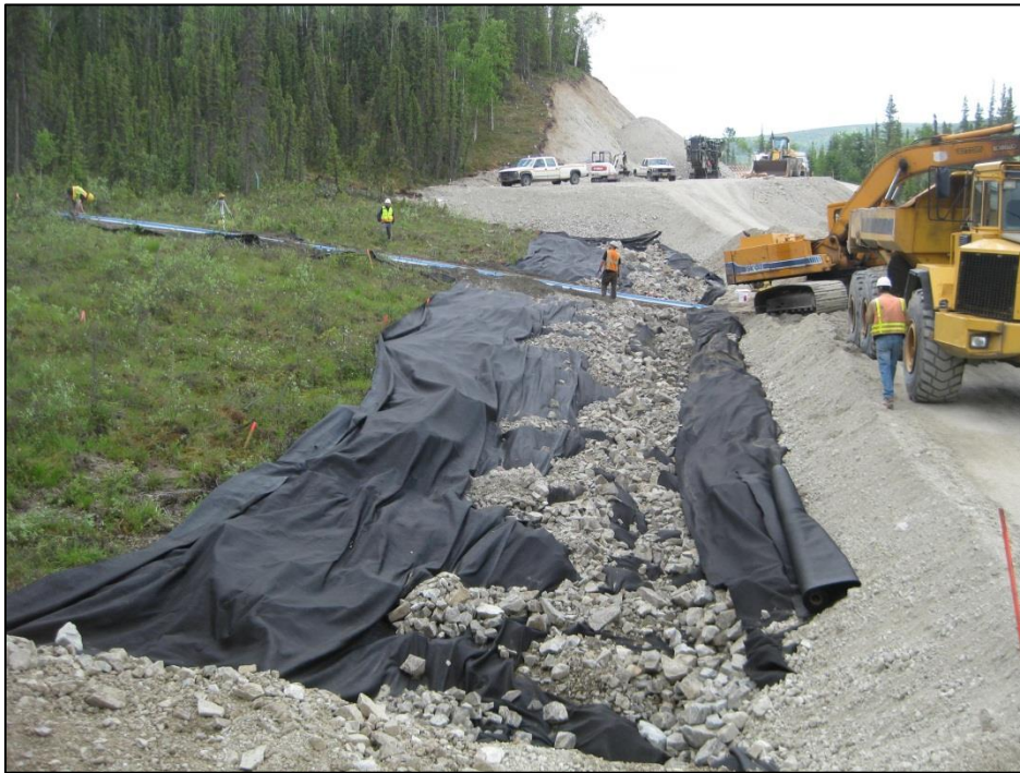
Figure C-1. Looking southeast towards the instrumented cross section. Geotextile with some ACE material is present in the foreground. (Photograph by M. Darrow, June 2012)
