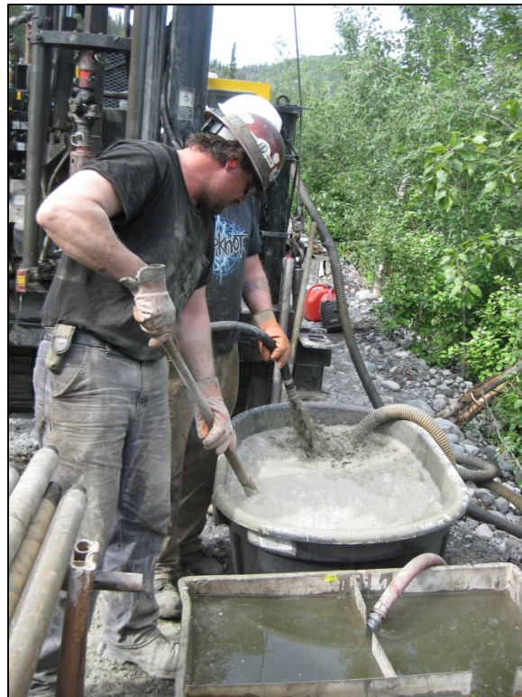
Figure B-6. Preparing the cement-bentonite grout for backfill into TH10-1553. (Photograph by M. Darrow, June 2010)
