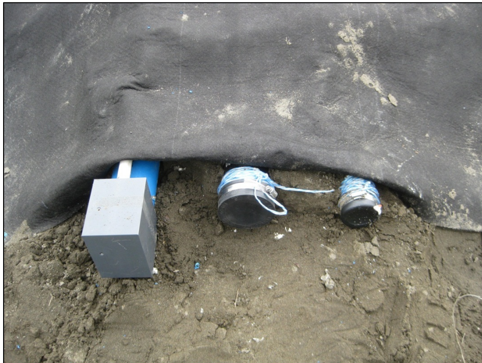
Figure C-17. Upslope casing ends secured. From left to right, dead-end pulley on guide casing for manual inclinometer probe measurements, sealed guide casing with tied-off SAA pull rope, sealed 2-in. PVC casing with tied-off TAC/thermistor string pull rope. (Photograph by M. Darrow, July 2012)
