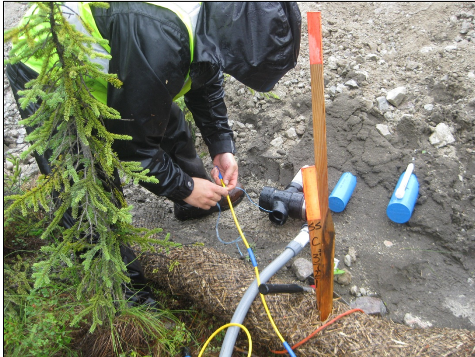
Figure C-7. Attaching the pull rope to the end of the TAC device. (Photograph by M. Darrow, July 2012)
