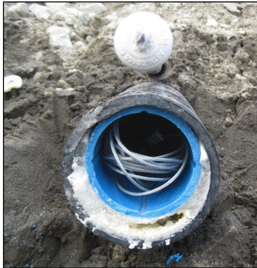
Figure C-23. Downslope guide casing termination. Wire rope is tucked into casing for easy retrieval for next reading. (Photographs by M. Darrow, July 2012)
