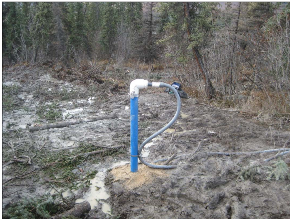
Figure D-6. Completed casing and instrument installation in TH12-9004. (Photograph by M. Darrow, Sept. 2012)
