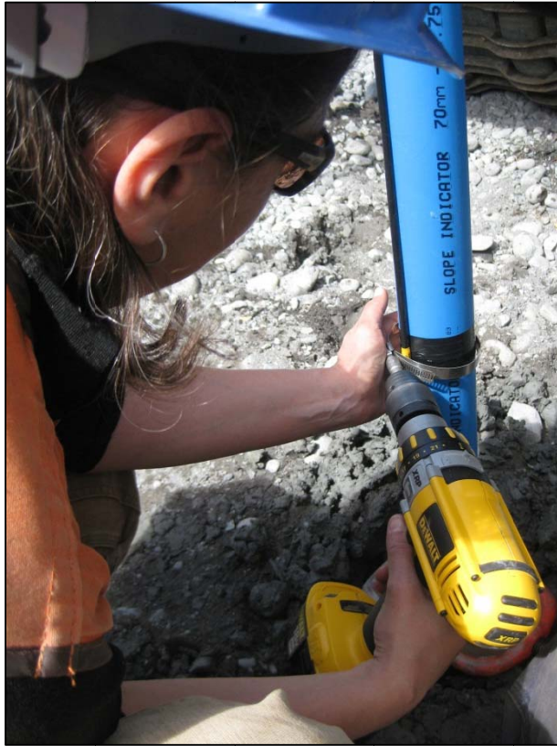
Figure B-3. Attaching the coaxial (TDR) cable with hose clamps at 10-ft intervals. (Photograph courtesy of T. Haller, June 2010)
