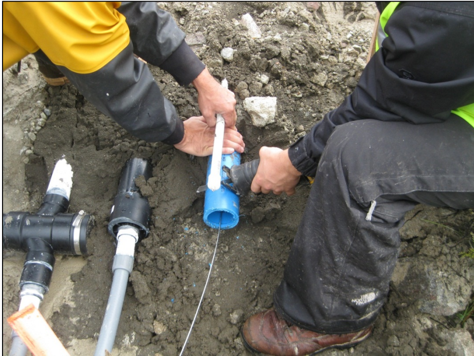
Figure C-18. Trimming the downslope guide casing for ABS end cap adapter. (Photograph by M. Darrow, July 2012)
