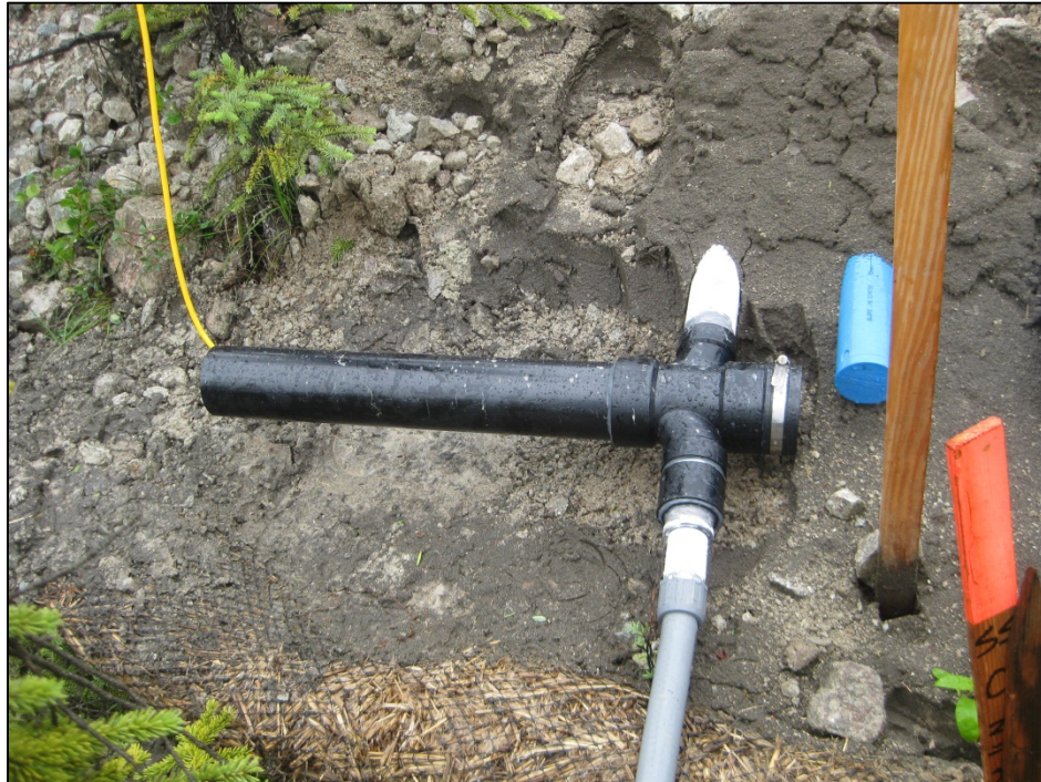
Figure C-9. PVC casing to flexible conduit adapter for the temperature measurement cables. (Photograph by M. Darrow, July 2012)
