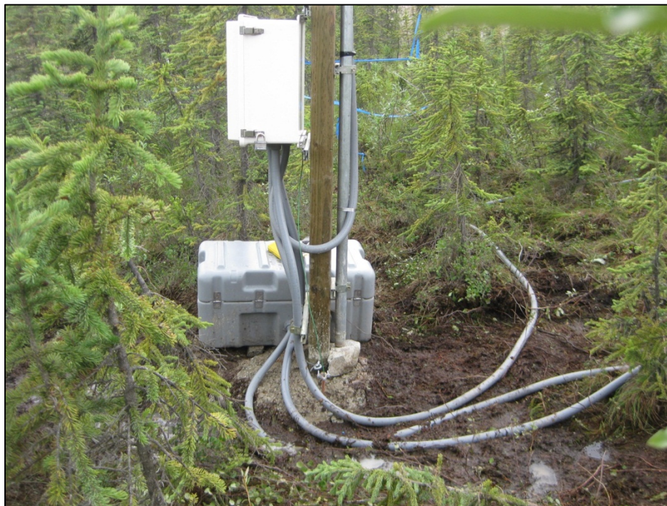
Figure C-25. Battery box and enclosure for ADAS. (Photograph by M. Darrow, July 2012)
