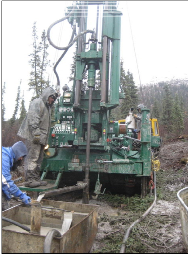
Figure D-1. Drilling TH12-9004 with tricone and casing. (Photograph by M. Darrow, Sept. 2012)
