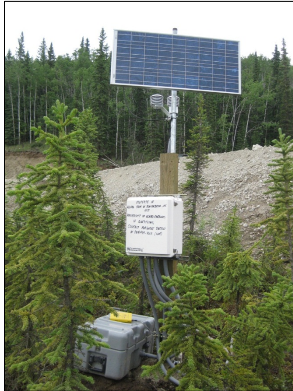
Figure C-26. Final ADAS configuration located near the downslope toe of the embankment. The thermal berm is visible behind the ADAS. (Photograph by M. Darrow, July 2012)
