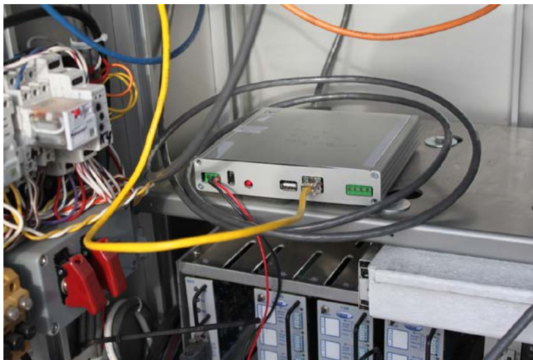
Figure 3.17: Snapshot of DCU Installed in Intersection Lynn Ave & TH 13
