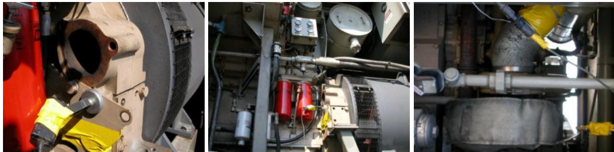
Figure 3-13. Installation of Sensors on a GP40 Locomotive Head End Power Engine (a) engine RPM sensor (front view), (b) engine RPM sensor (side view); (c) intake air temperature (IAT) sensor
