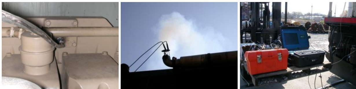
Figure 3-14. Installation of PEMS Exhaust Sample Lines in a GP40 Locomotive (a) MAP sampling hose on the HEP engine; (b) sampling hose on HEP engine exhaust; (c) PEMS main unit on forklift next to locomotive
