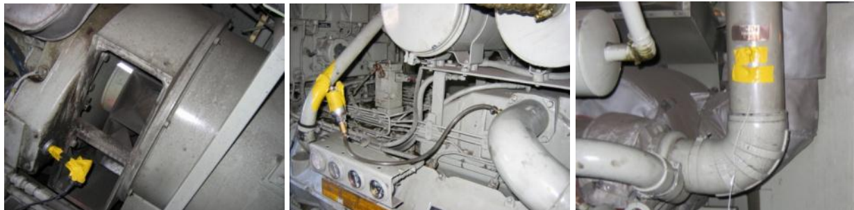
Figure 3-9. Installation of Sensors on an F59PHI Locomotive Head End Power Engine (a) engine RPM sensor; (b) manifold absolute pressure (MAP) sensor; (c) intake air temperature (IAT) sensor
