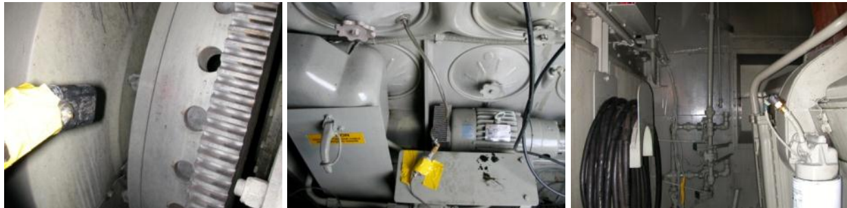
Figure 3-8. Installation of Sensors on an F59PHI Locomotive Prime Mover Engine (a) engine RPM sensor; (b) manifold absolute pressure (MAP) sensor; (c) intake air temperature (IAT) sensor
