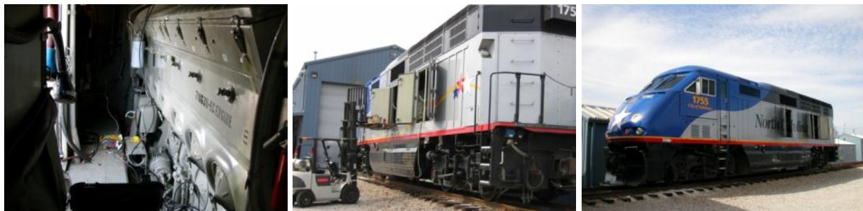
Figure 3-10. Installation of PEMS Exhaust Sample Lines in an F59PHI Locomotive (a) routing sampling hoses and cables; (b) routing sampling hoses through a side door, secured with ties (rear-view); (c) side-view of F59PHI locomotive
