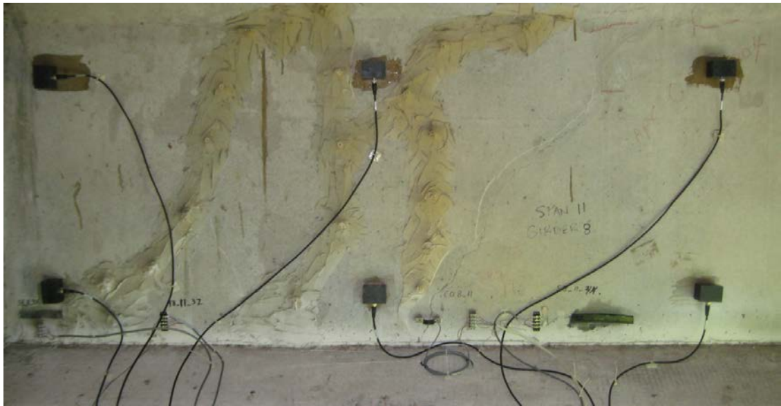
Figure 4-8: Arrangement of Sensors 13-18 on Girder 8
