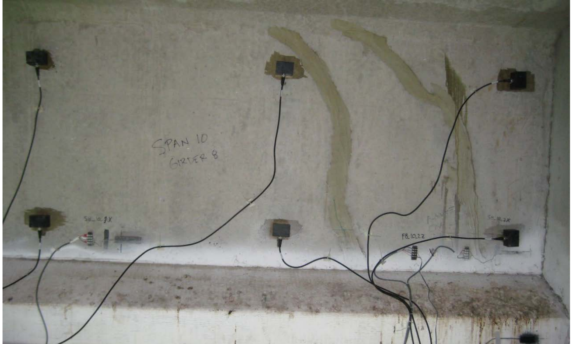
Figure D-4: Visible cracks on face of SP10G8
