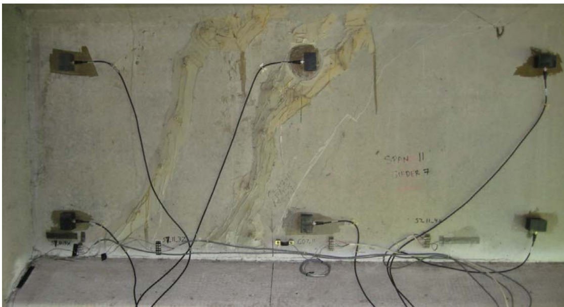
Figure 4-10: Arrangement of Sensors 19-24 on Girder 7
