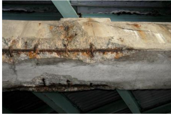
Figure 3-17: Corrosion of steel reinforcing bars in concrete (Courtesy of Matco Services, Inc.).
