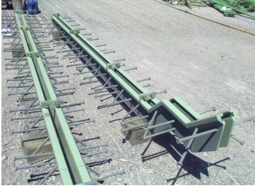
Figure 2-4: New dam hardware
