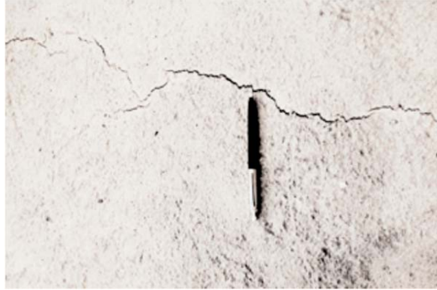
Figure 1-3: Plastic shrinkage crack in concrete slab (photo from PCA 2011)
