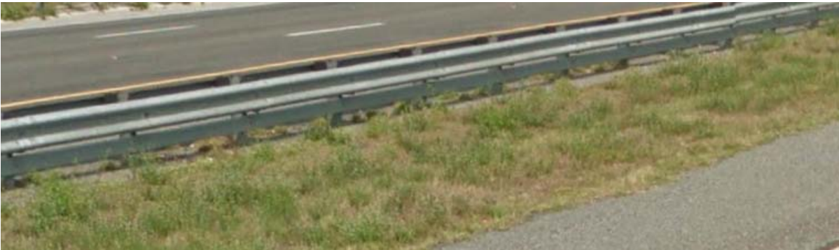
Figure 1-2: G4 (1S) Strong-post W-beam Guardrail with a Rub-rail on I-95 in St. Johns County
