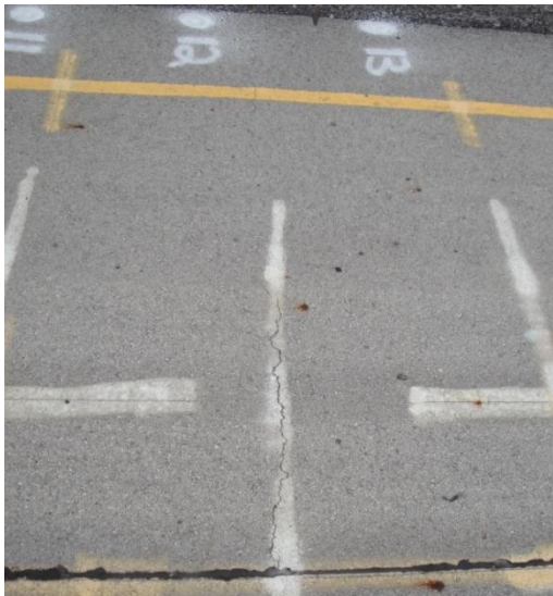
a) Initiation of reflection cracking
