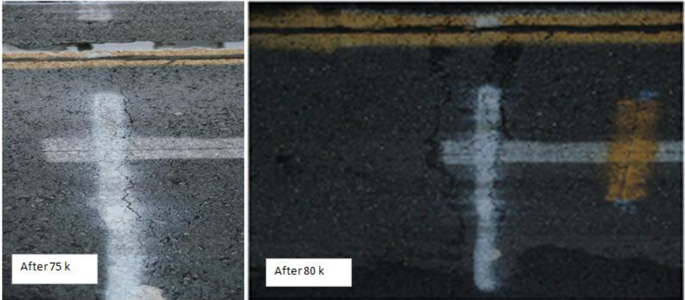
Figure F-5. Reflective Cracking on Control Section 4 (Type C; 4.3% OAC = 50% LTE. (For Section 3_Control (Type C; 4.3% OAC) = Good LTE; cracks appeared only after 175 k ALF load passes)
