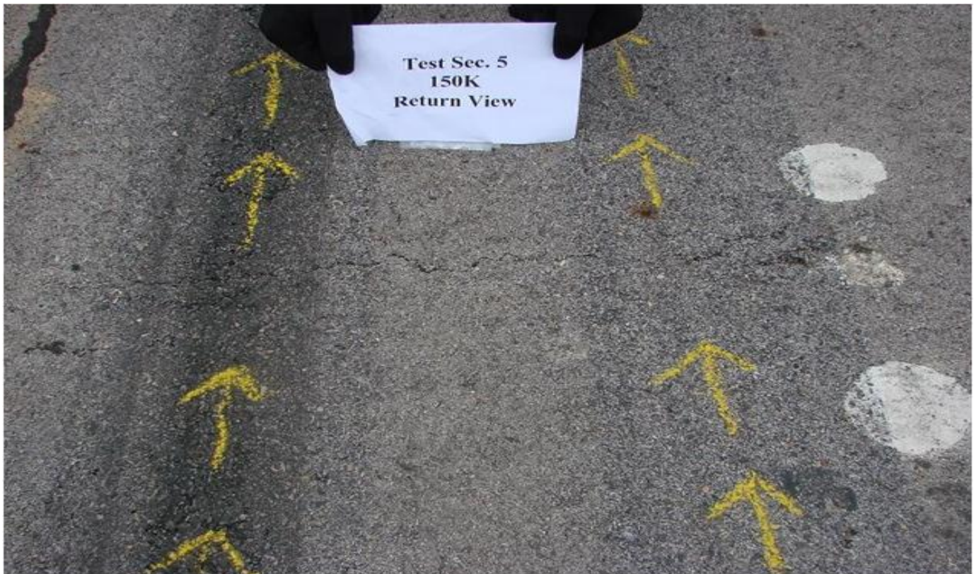
Figure F-6. Section 5 _Modified (Type C; 5.2% OAC) = Good LTE; Cracking at Joint Location Station# 47.5 after 143 k ALF Load Passes
