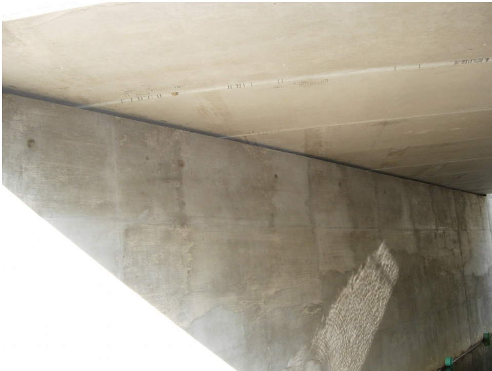
Figure 5-7 View of the Bottom Surface and West Abutment of the Knoxville, MD, Bridge
