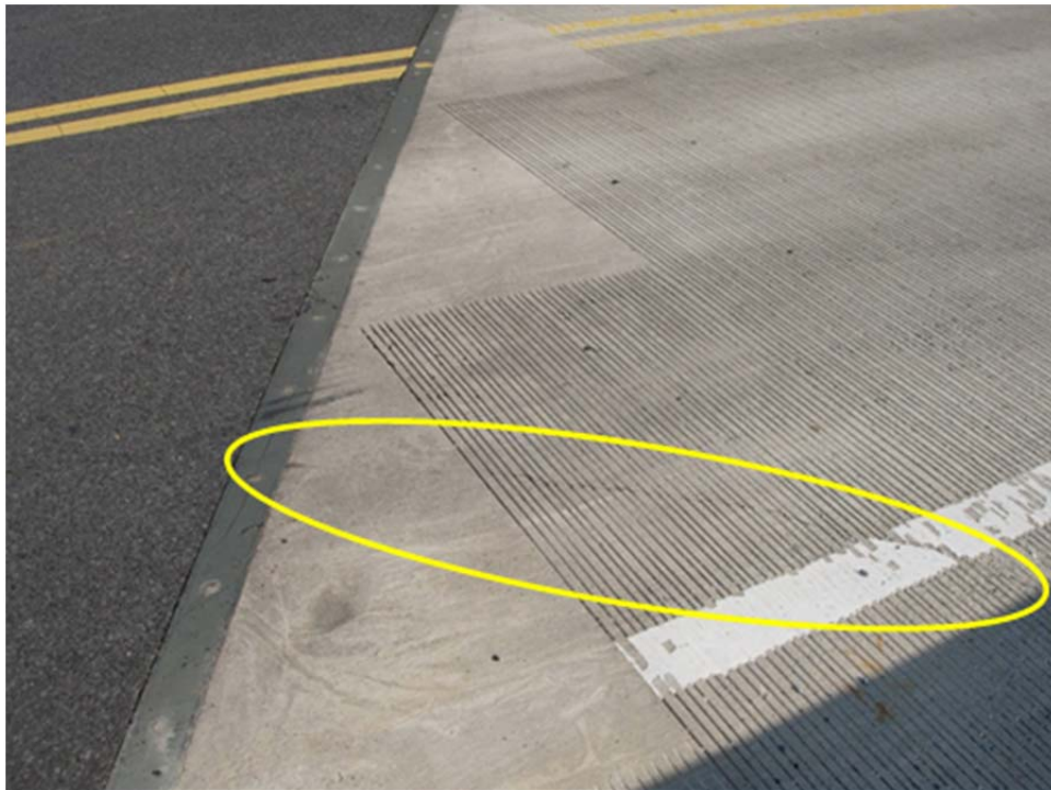
Figure 5-5 Longitudinal Crack on the Top Surface of the Knoxville, MD, Bridge
