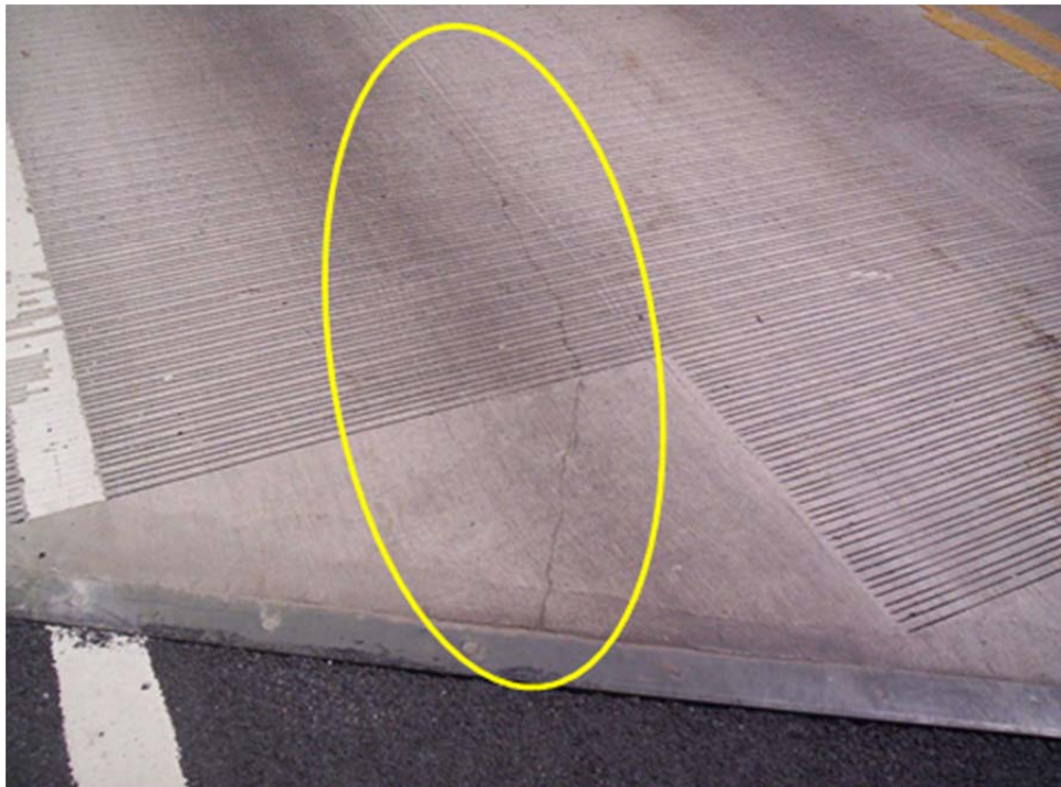
Figure 5-3 Longitudinal Crack on the Top Surface of the Knoxville, MD, Bridge
