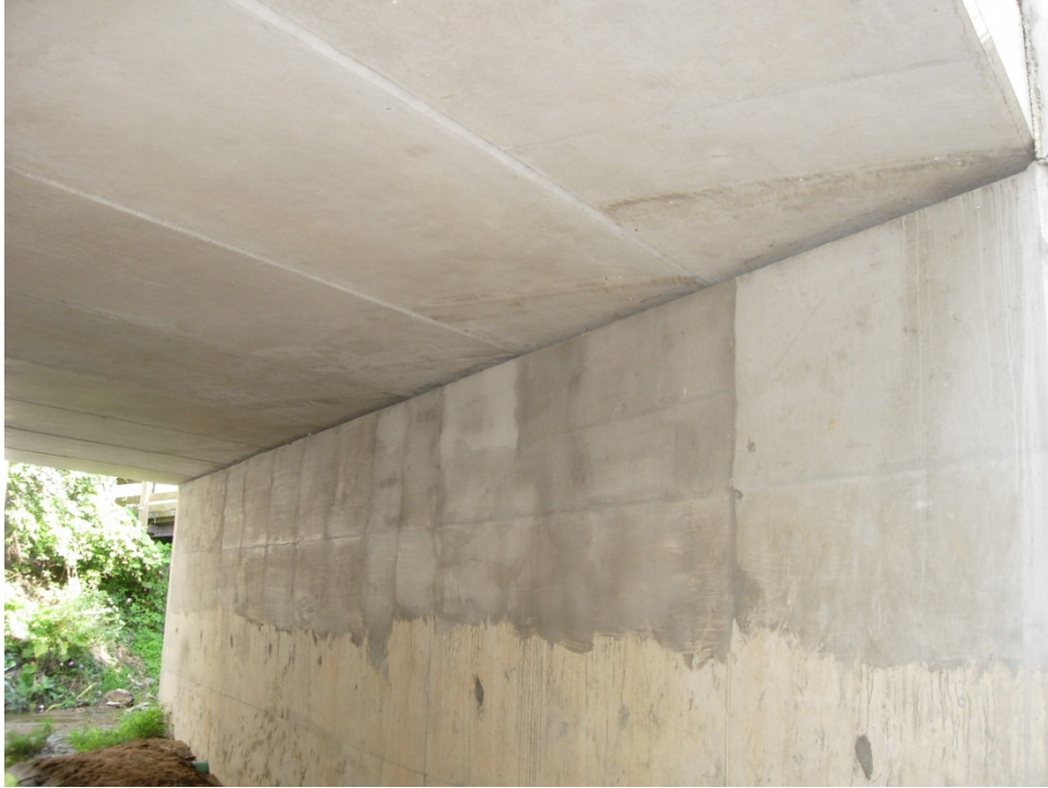
Figure 5-6 View of the Bottom Surface and the East Abutment of the Knoxville, MD, Bridge
