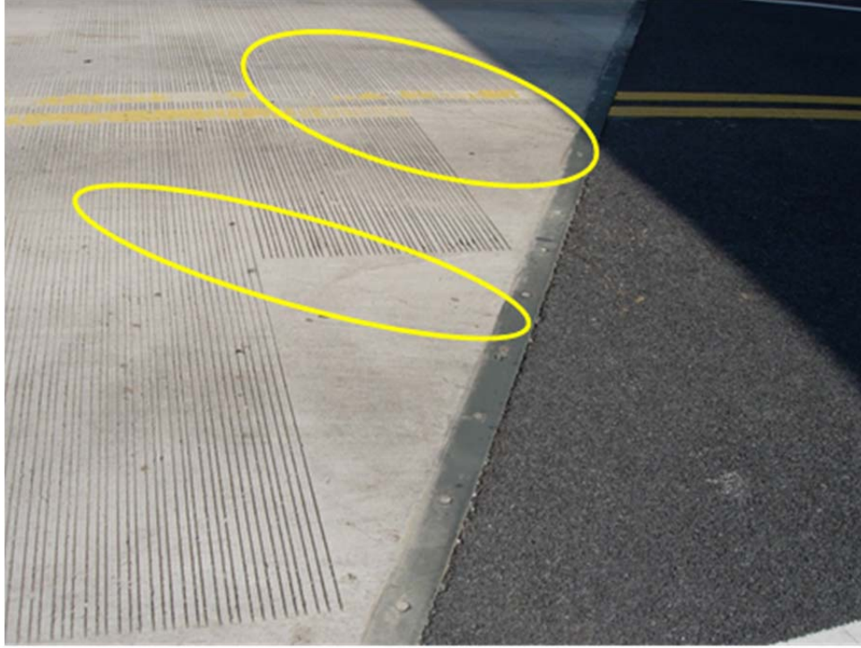
Figure 5-4 Longitudinal Cracks on the Top Surface of the Knoxville, MD, Bridge
