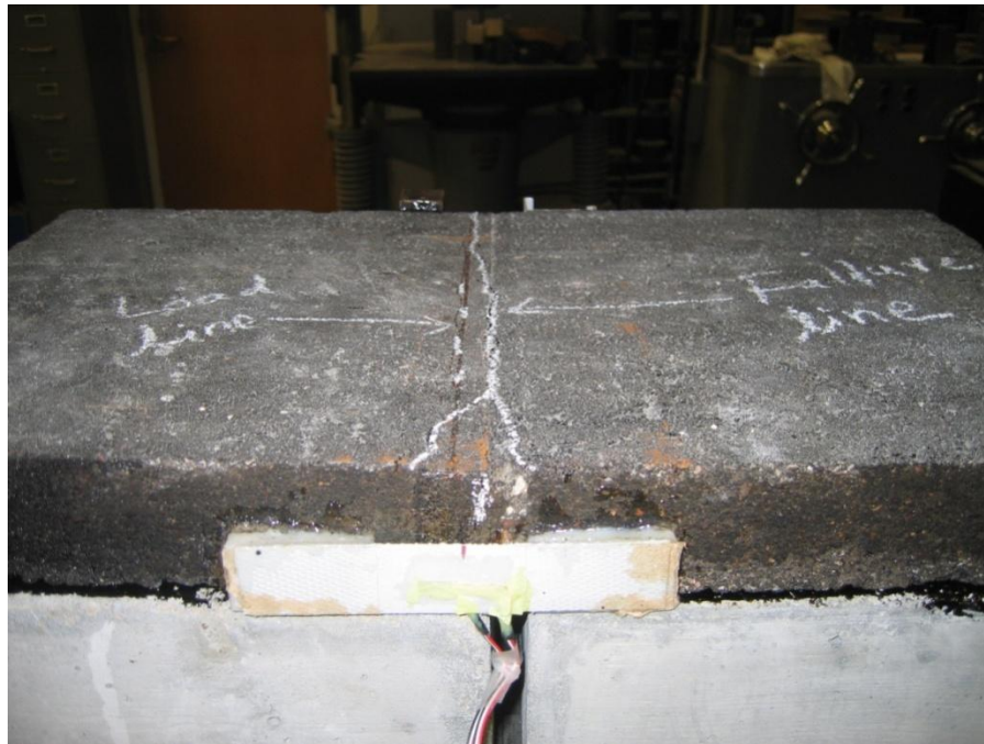
(a) Cracks on top of the HMA overlay
