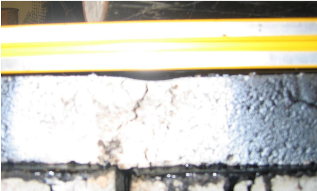
FIGURE 4.15 Crack Initiated Due to Shear from the Top of the HMA Overlay
