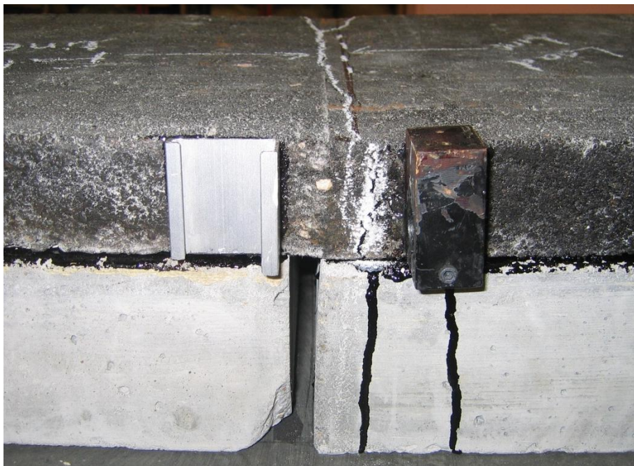
(b) Cracks on one side of the HMA overlay
