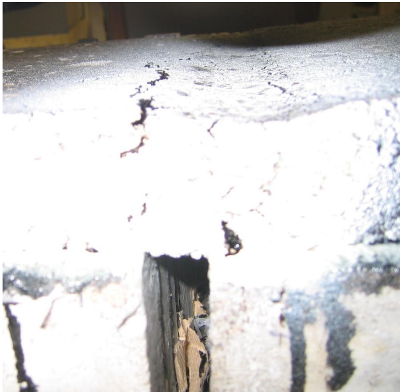
FIGURE 4.14 Crack Initiated Due to Bending from the Top of the HMA Overlay
