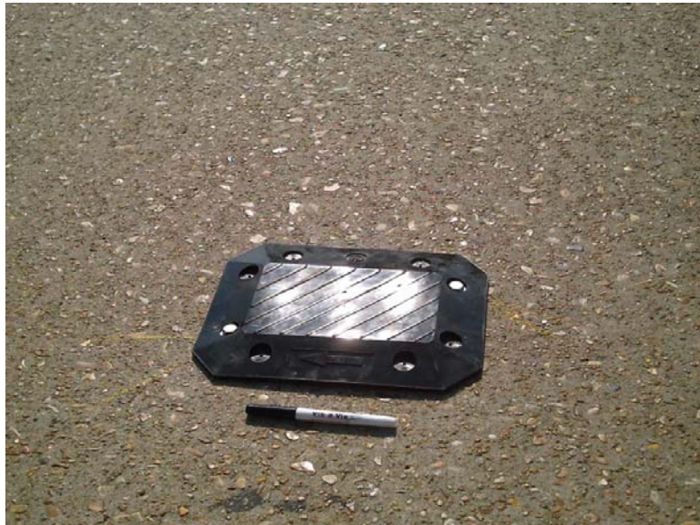
Figure 13 Attached MIR with protective cover
