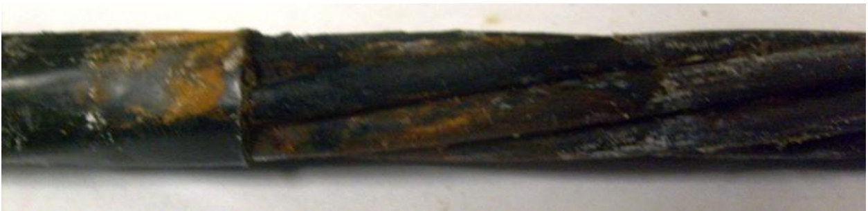
FIGURE 9d Specimen G/SFG-1, 15 Weeks, after Removal of Grout. Close-up on Strand in Gypsum Grout
