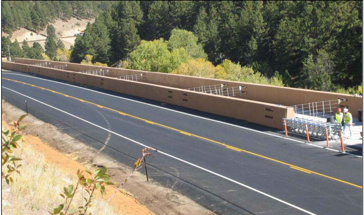
Figure 4.4 The novel ramp design on Wyoming Highway 14, in the eastbound lane just outside of Buffalo. The older ramp was on the other side of the highway, requiring the driver to cross oncoming traffic. The metal mesh webs are designed to absorb energy to a point and then break away.
