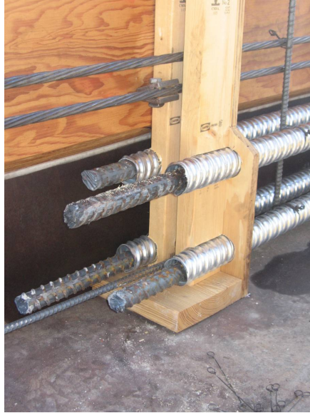
Figure 10.4. Unstressed reinforcing bars placed in ducts to keep ducts straight during placing of concrete
