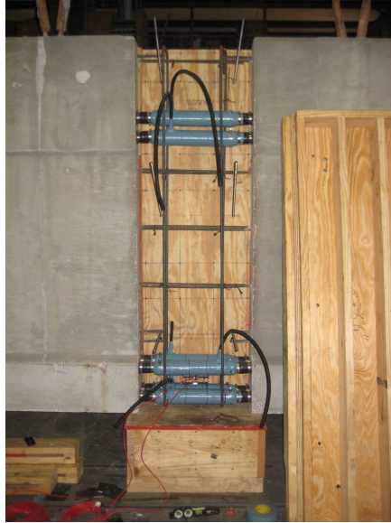
Figure 10.9. Duct couplers in closure strips, sealed with tape prior to concrete placement
