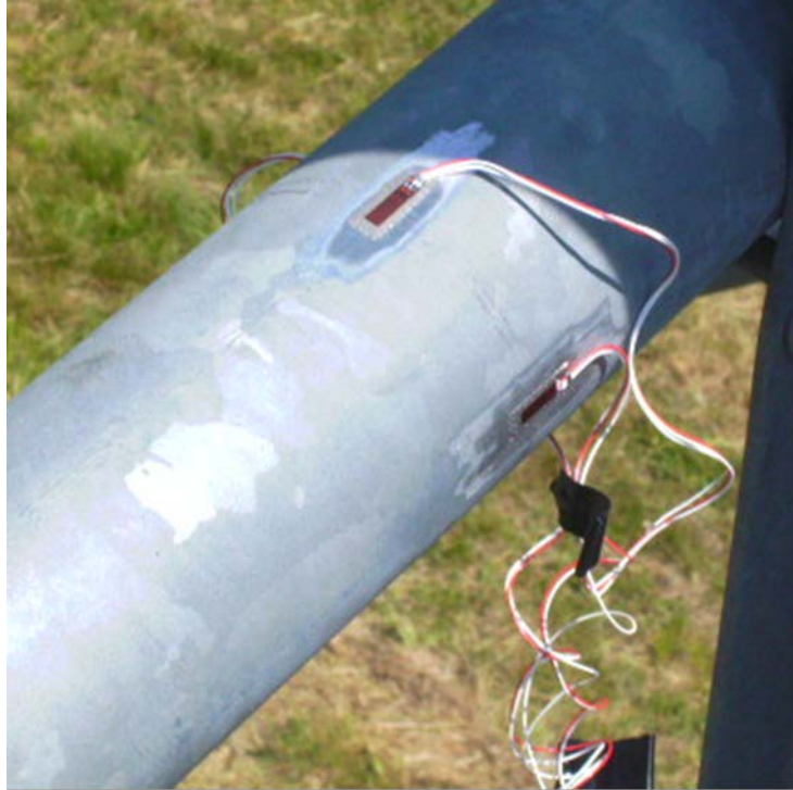
Figure 5-5. Uncovered uni-axial strain gauges attached to the truss chord member at location 3
