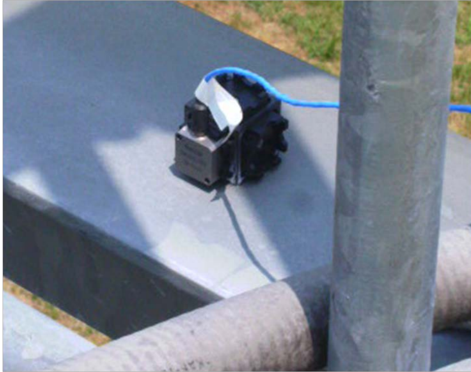
Figure 5-11. Accelerometer 1L measuring the upright in the longitudinal direction normal to traffic
