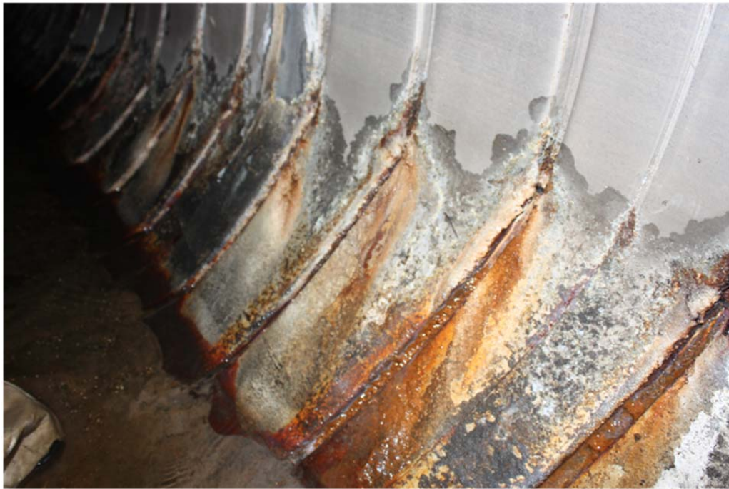
Figure 7: Photograph of in-situ pipe located in Jacksonville, near Highland Glen and Beach Blvd. Mechanical damage (top left, bottom), Limestone rocks present beneath the bore location (top right).
