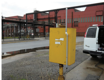
(f) Other roadside electrical equipment.
