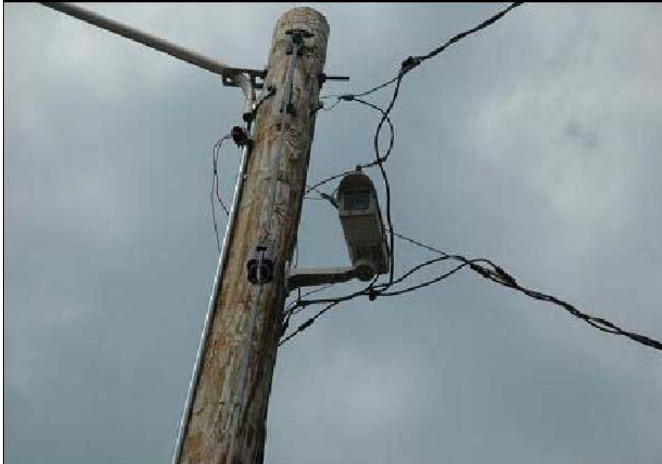
Figure 3.3 Camera Installed at HRGC to Capture Crossing Maneuvers
