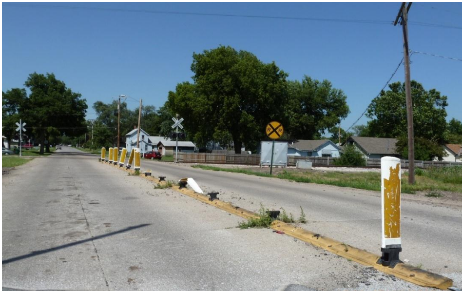
Figure 3.6 Dilapidated Condition of Barrier at Fremont due to Lack of Maintenance
